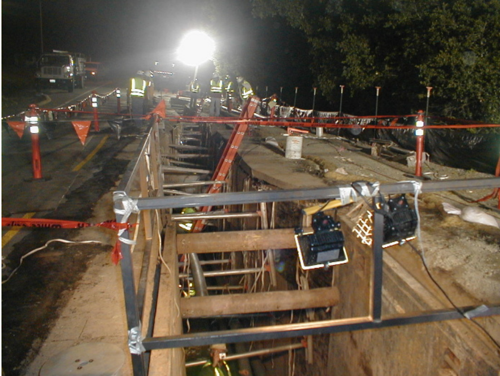
Figure 1 – Trenching activities south of Manhole #20 in Caltrans right-of-way on Skyline Boulevard, Segment 1, May 23, 2005
