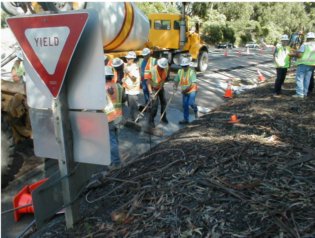
Figure 2 – Cement slurry spill in trenching area between Manholes #36 and #37 on Skyline Boulevard, Segment 2 Underground, May 25, 2005
