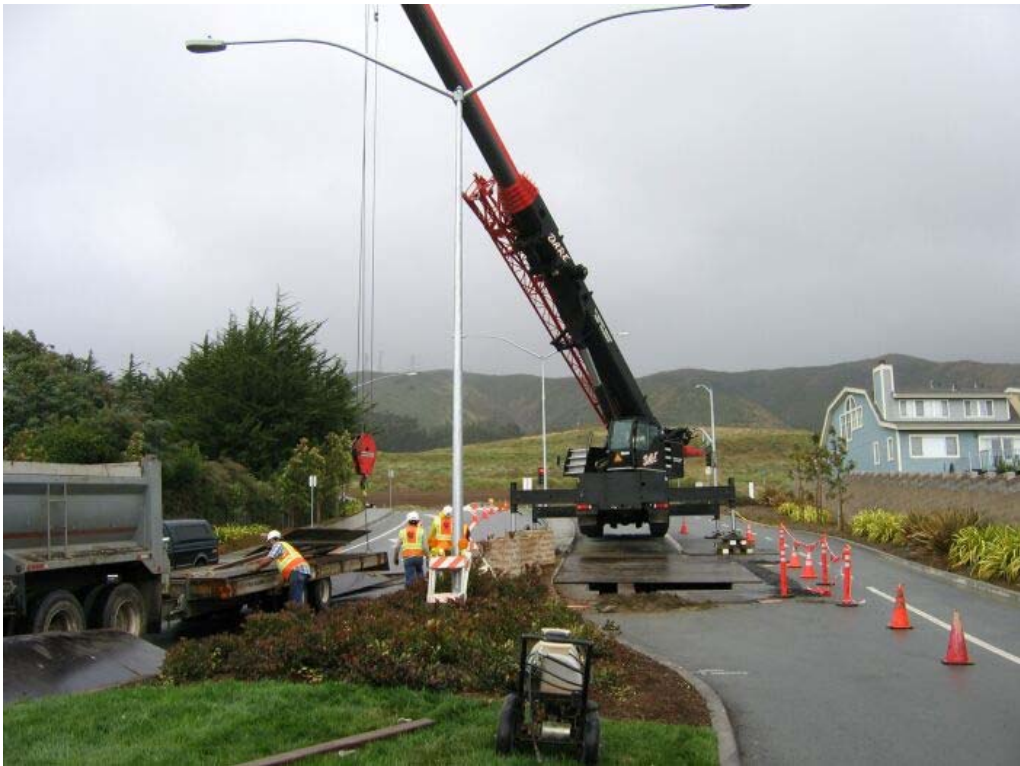
Figure 4 – Crews plating Manhole #58 pit after vault was set on Lawndale Drive, Segment 4, June 16, 2005.
