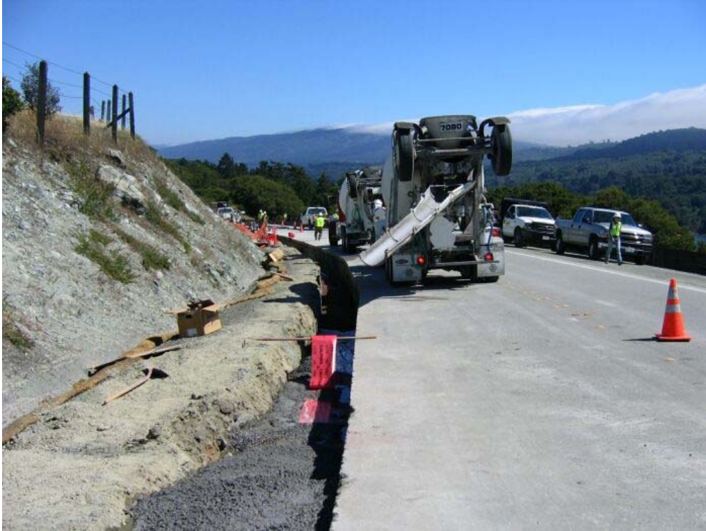
Figure 1 – Cement slurry being poured over installed conduit in trench between Manholes #23 and #24, Segment 1, June 28, 2005
