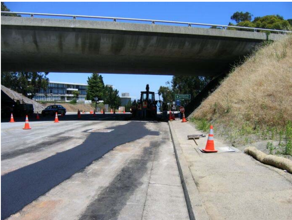
Figure 2 – Communication box set and trench paved on Trousdale Drive, Segment 2 Underground, July 1, 2005
