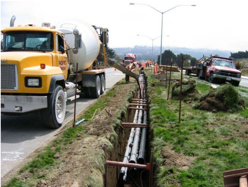
Figure 4 – Pouring cement slurry over installed conduit in trench in median along Lawndale Drive in the Town of Colma, Segment 4, June 28, 2005.
