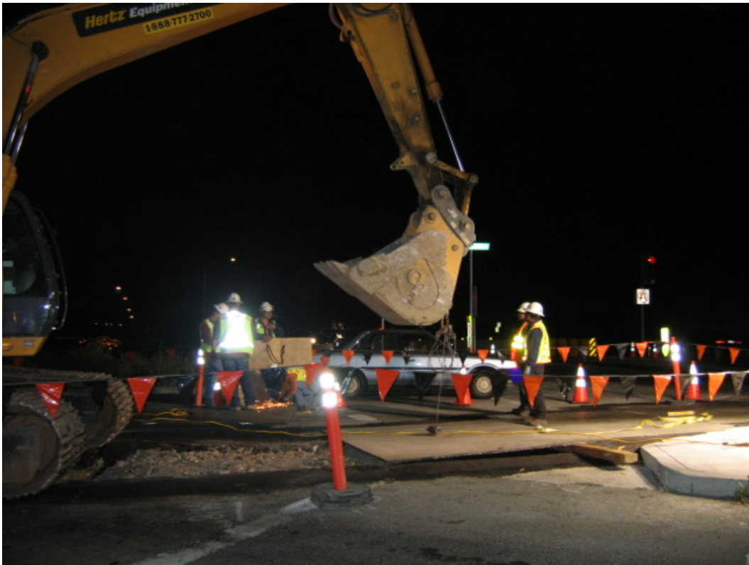
Figure 5- Night work at the intersection of Bayshore Boulevard and Guadalupe Canyon Parkway in the City of Brisbane, Segment 5, June 28, 2005
