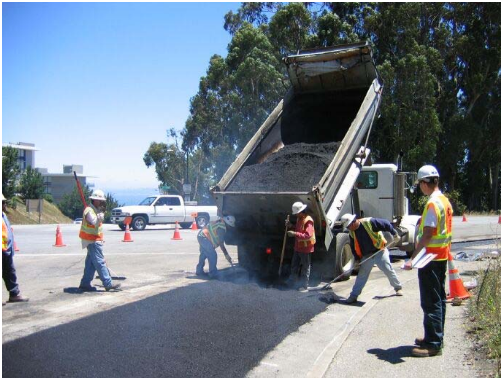
Figure 2 – Crews paving on corner of Trousdale Drive and Skyline Boulevard, Segment 2 Underground, July 8, 2005
