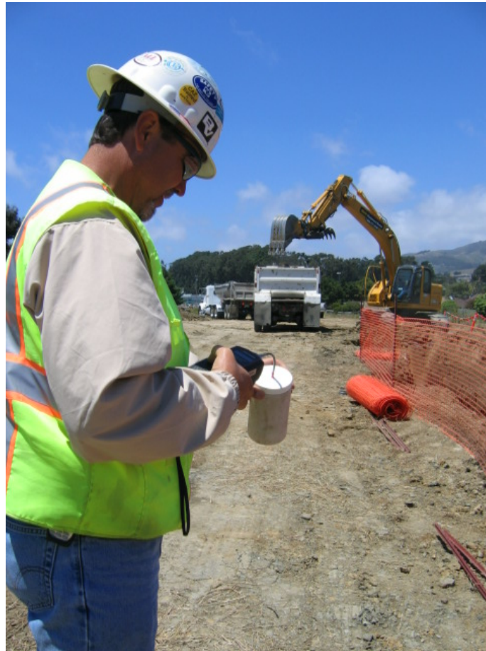
Figure 4 – Conducting soil monitoring test from trenched materia north of S. Spruce Street, Segment 4, July 8, 2005.
