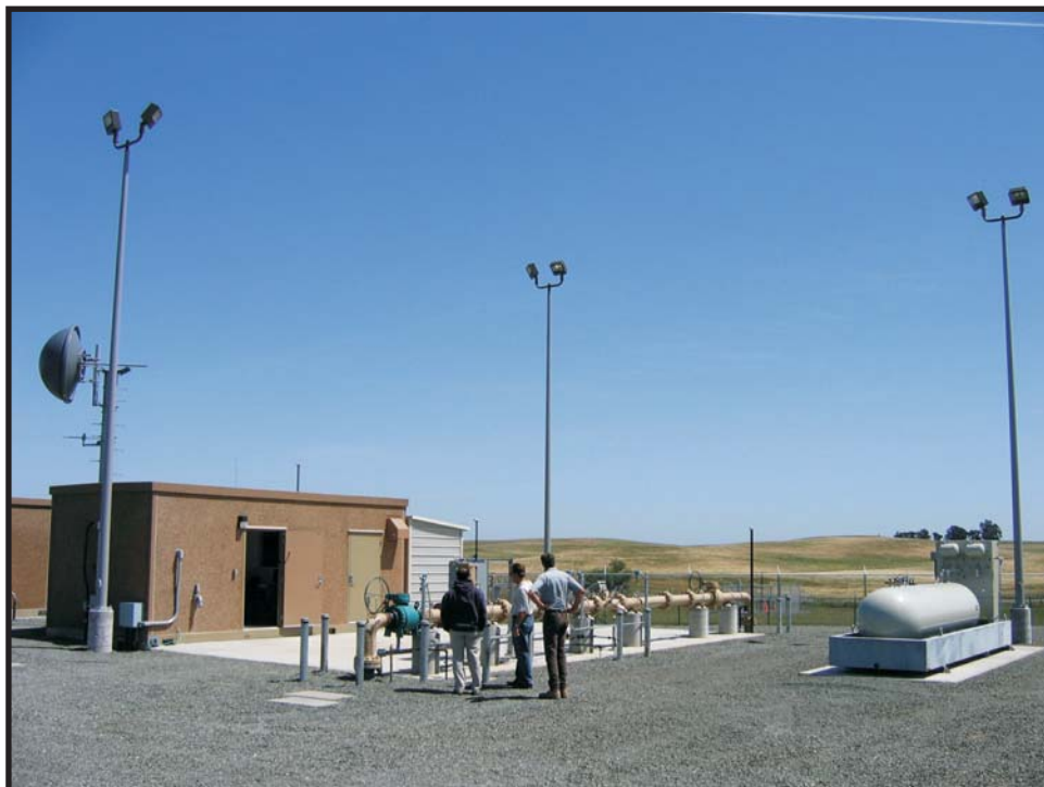
Metering Station constructed under the original Kirby Hills Natural Gas Storage Facility Project, April 26, 2007
