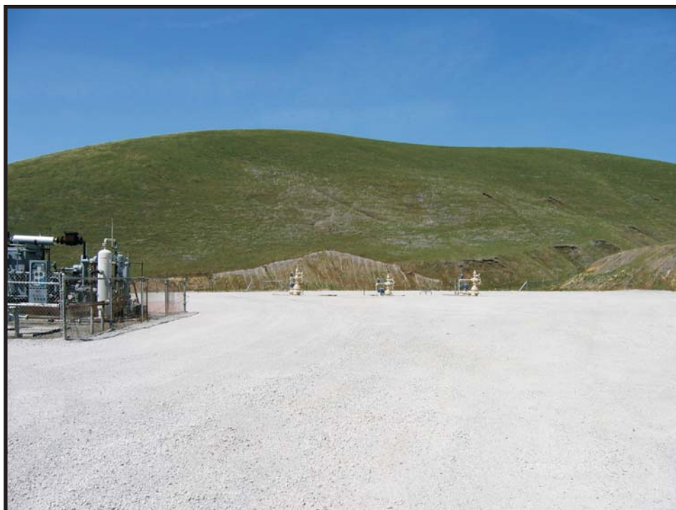
Well Site S-2 with three wells constructed as part of the original Kirby Hills Natural Gas Storage Facility Project, April 26, 2007
