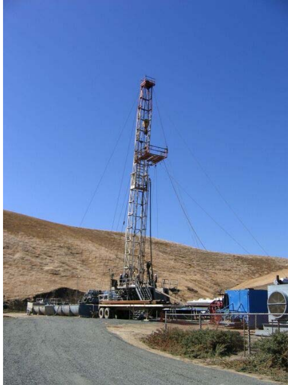
Figure 1 – Drilling rig set up at well site S-2 drilling well S2B, October 10, 2006.
