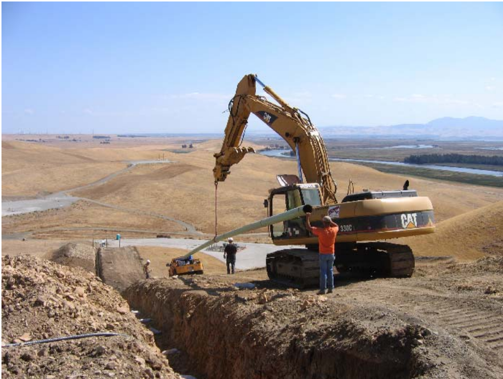
Figure 4 – Crews installing pipe in trench at top of hill near Well Site S-5. September 14, 2007.
