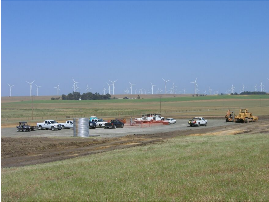
Figure 1 – Crews grading and moving soil from around the existing well pad at WS-22, May 6, 2008.
