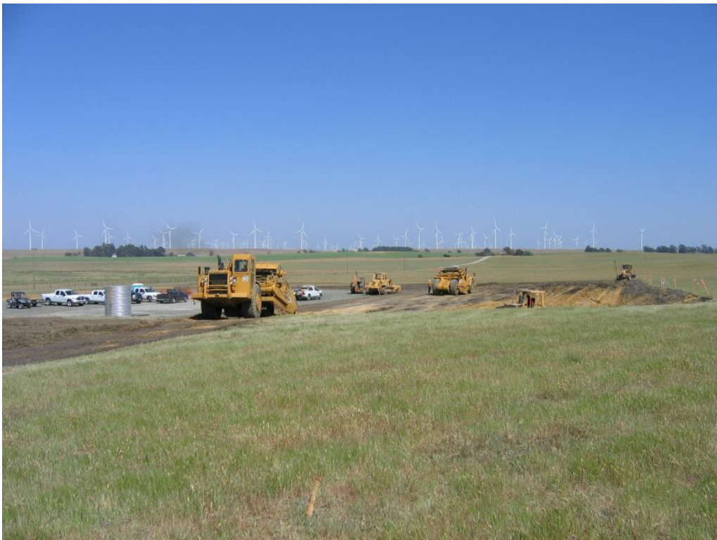
Figure 2 – Large earthmovers moving soil from WS-22 to WS-23 to build up well pad, May 6, 2008.
