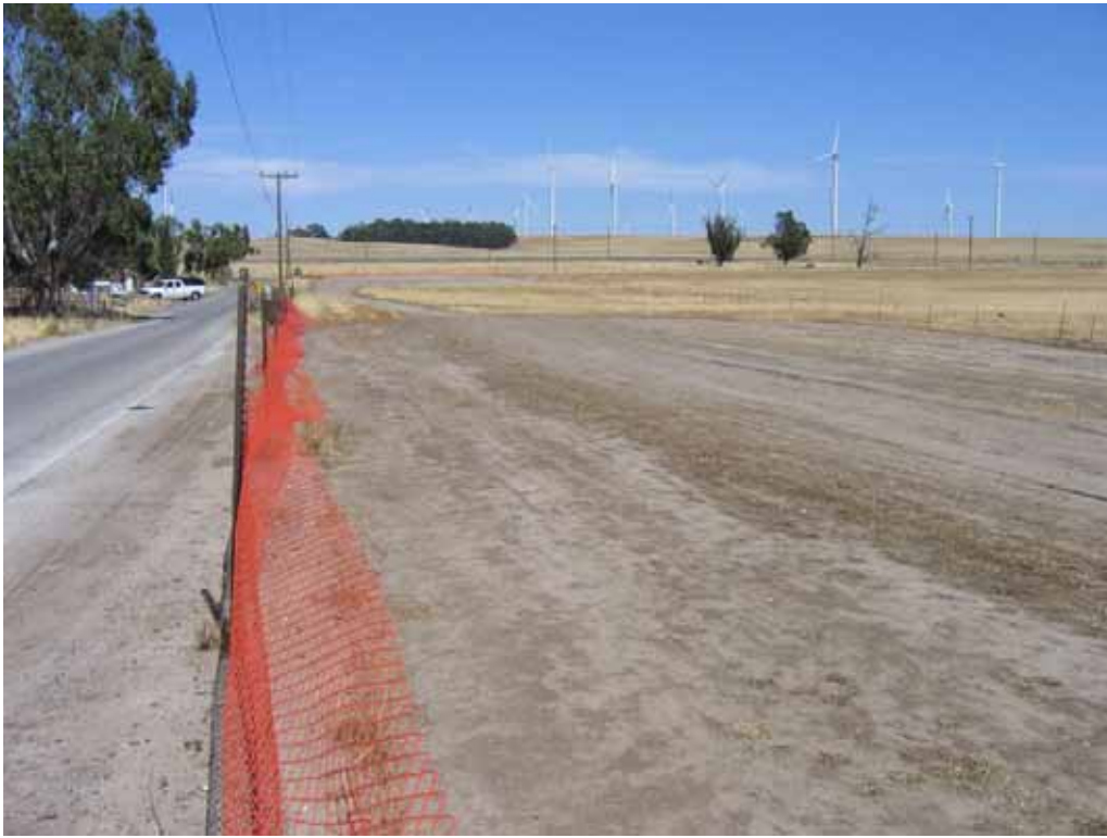
Figure 3 – Temporary access area west of Shiloh Road and south of the Kirby Hills access road cleared and compacted, June 20, 2008.
