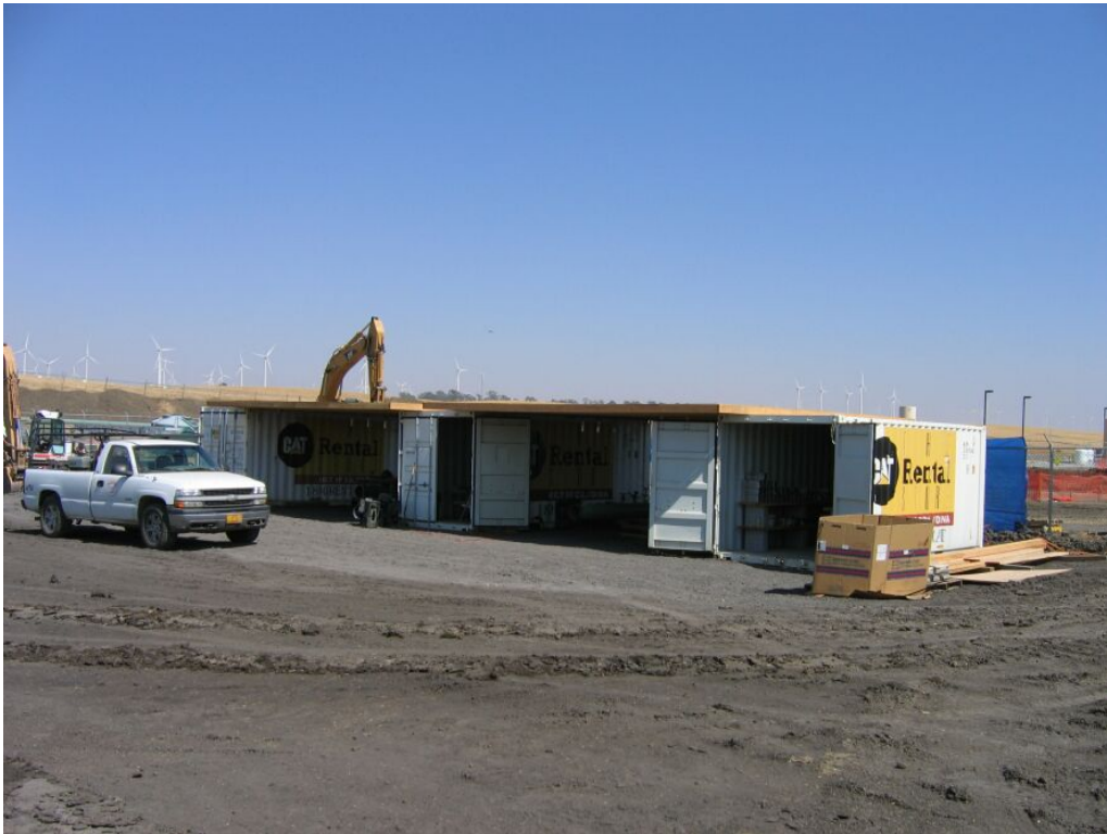
Figure 3 – Welder shack set up in temporary work area/staging yard on the north side of the Compressor Station, July 24, 2008.
