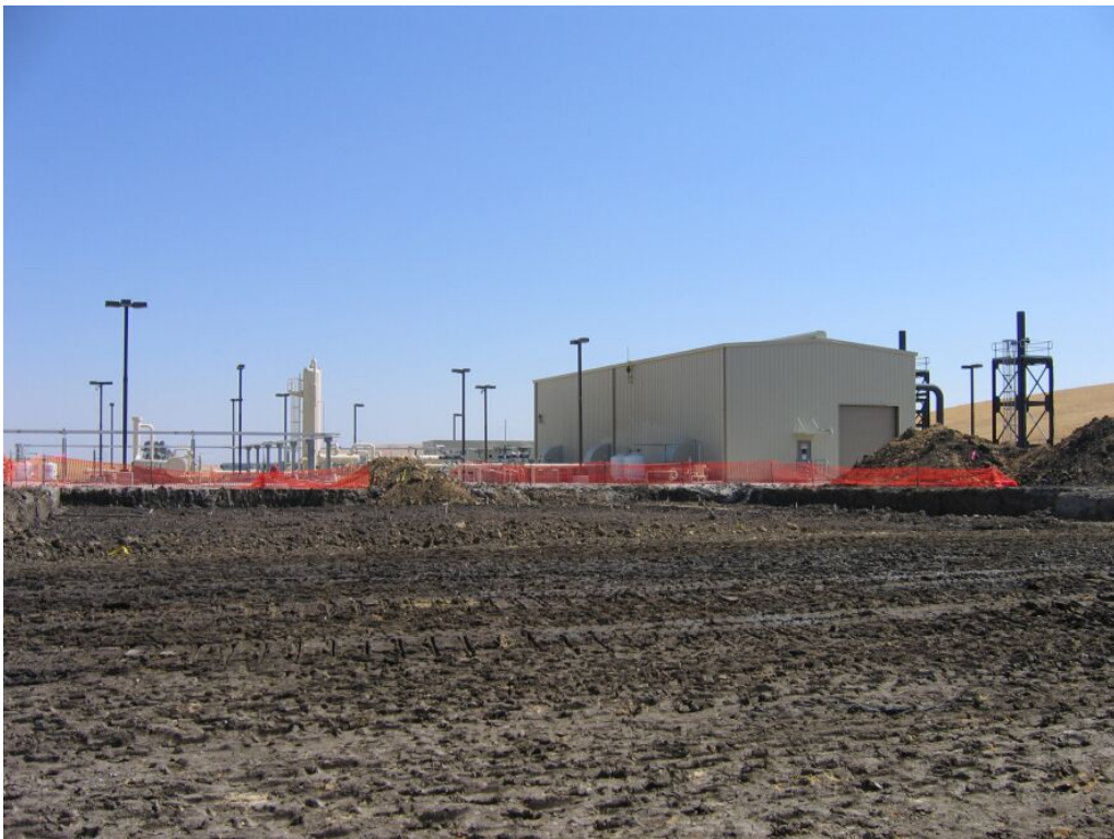
Figure 4 – Excavation for the new compressor building at the north end of the Compressor Station, July 24, 2008.
