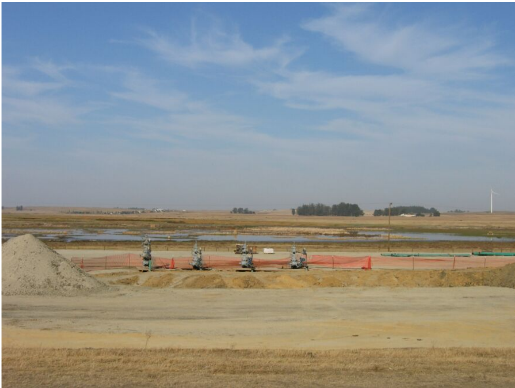
Figure 2 – Well heads at WS-22, October 17, 2008.
