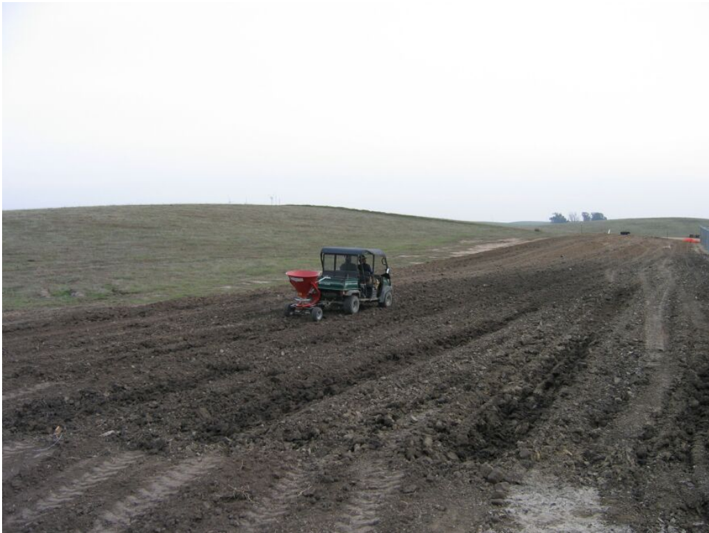
Figure 2 – Crews reseeding pipeline right-of-way on the east side of the compressor station, December 12, 2008.
