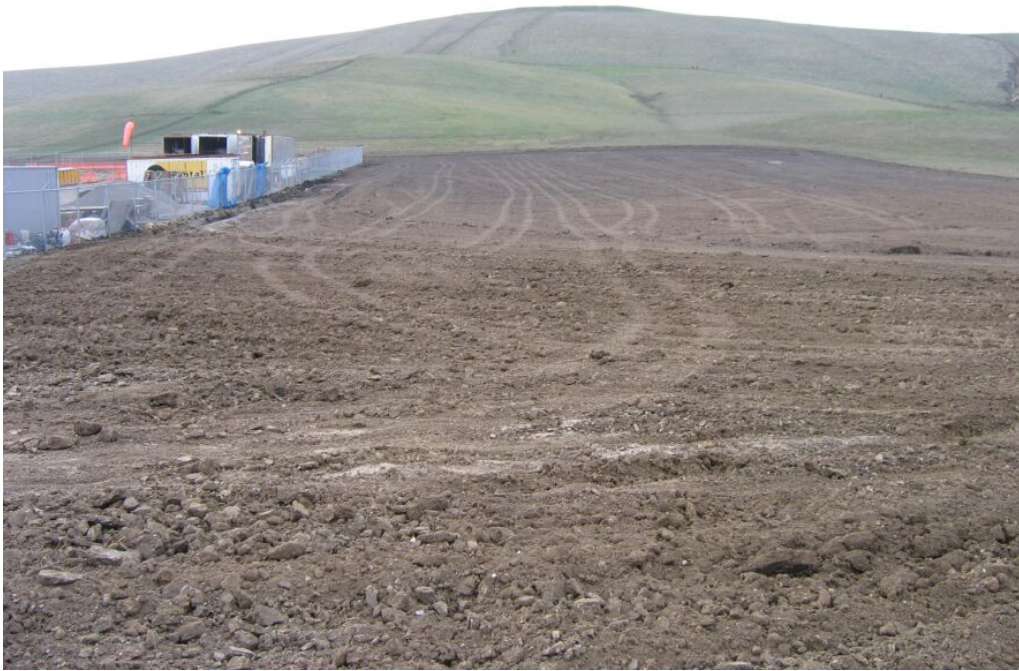
Figure 3 – Topsoil replaced over temporary work space/staging yard north of compressor station and the area reseeded, December 12, 2008.
