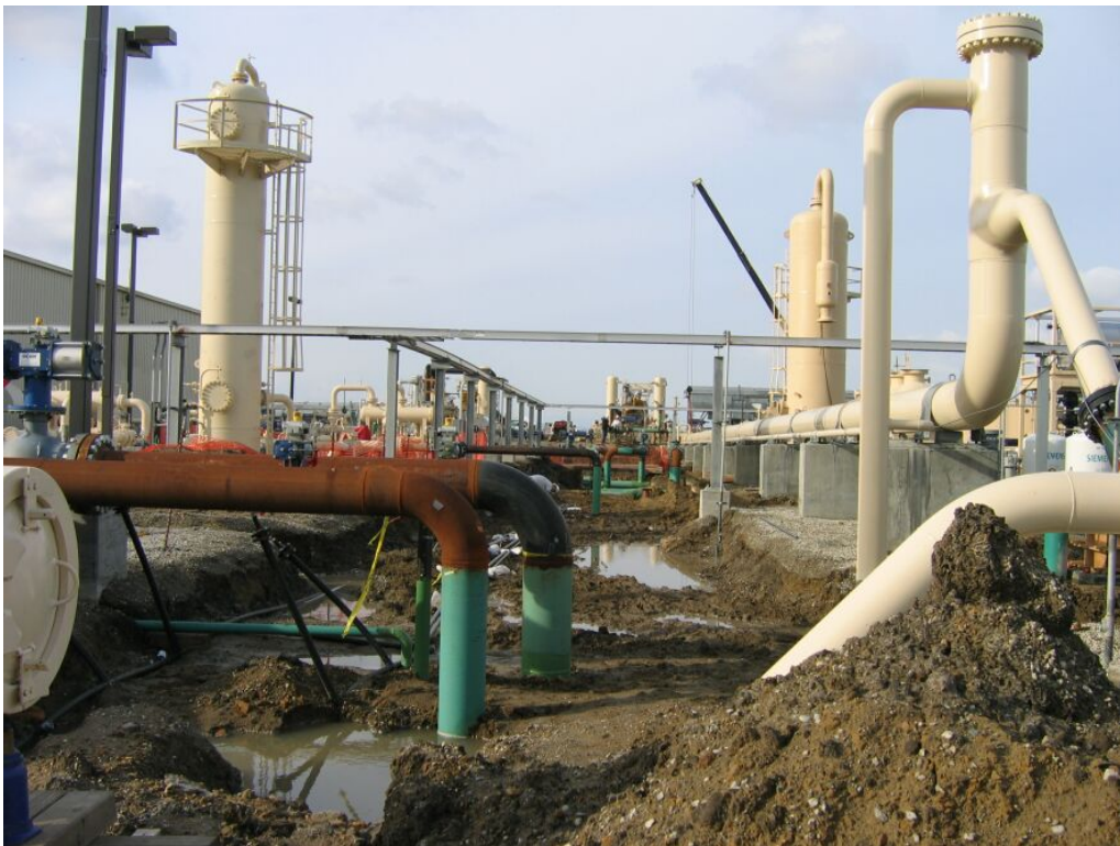
Figure 4 – Piping at the compressor station, February 18, 2009.
