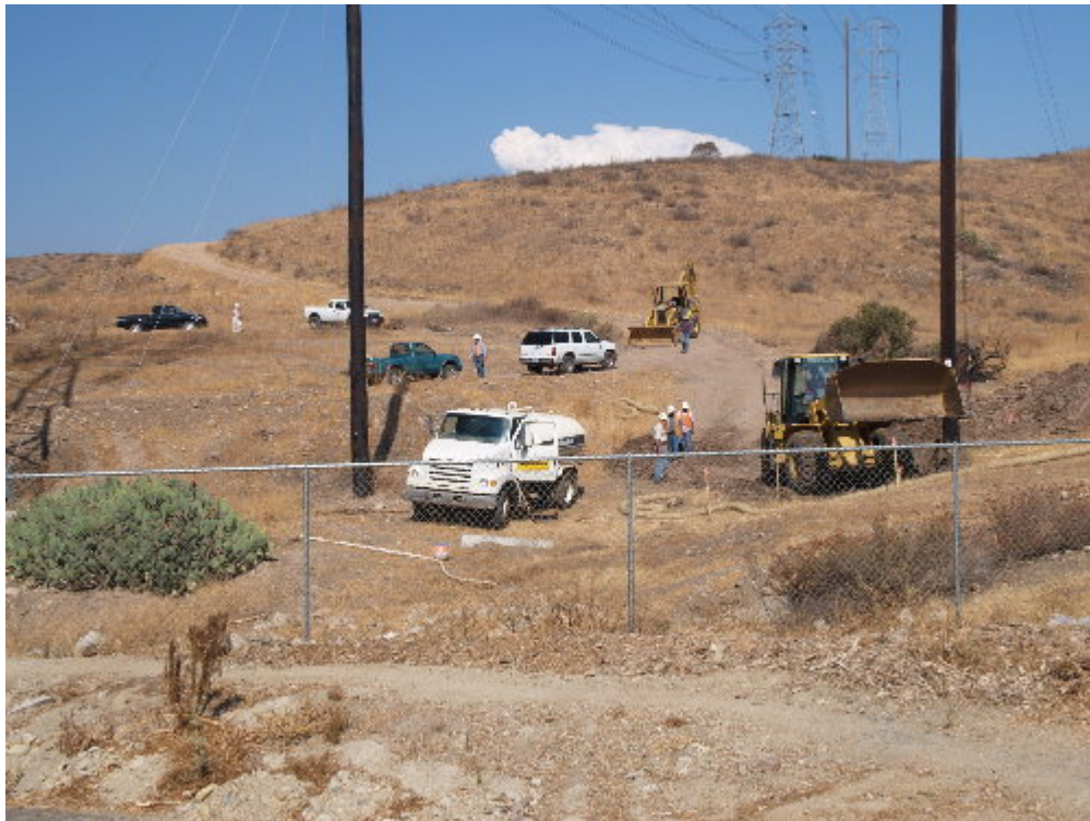
Figure 4 – Crew working on grading first pad. Water truck on-site for dust control.
