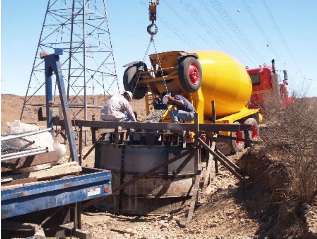
Figure 1 – The PAR crew at Tower Site 1340 prepared the forms and started the concrete pour.
