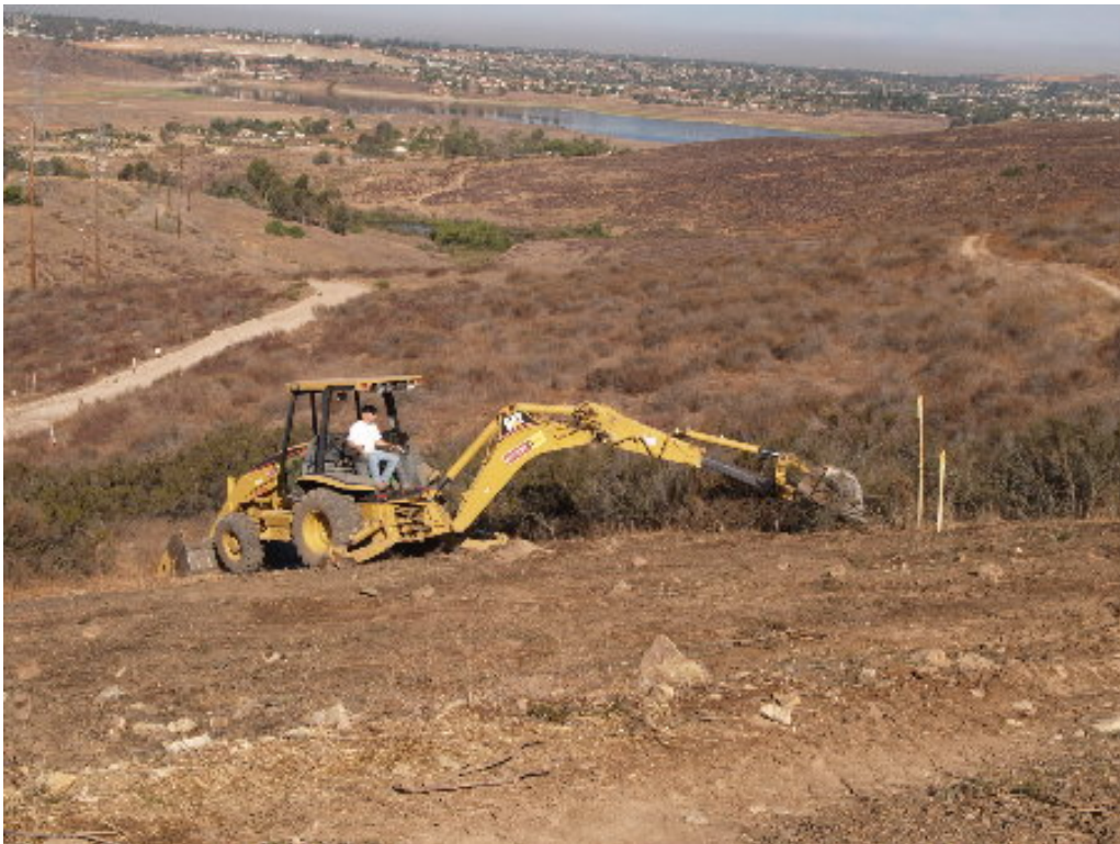
Figure 4 – The clearing crew worked with a backhoe to clear Tower 10 for grading.
