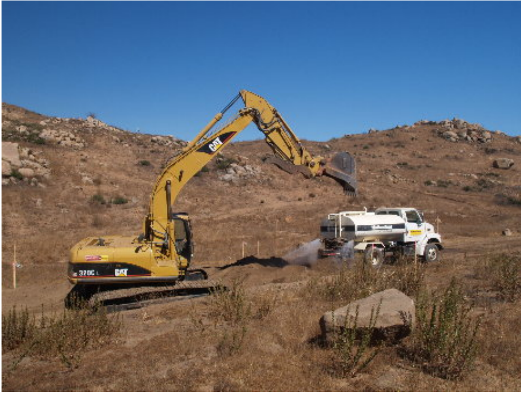
Figure 5 – The excavator operator and water truck driver worked to increase soil moisture prior to hauling to another site for fill.
