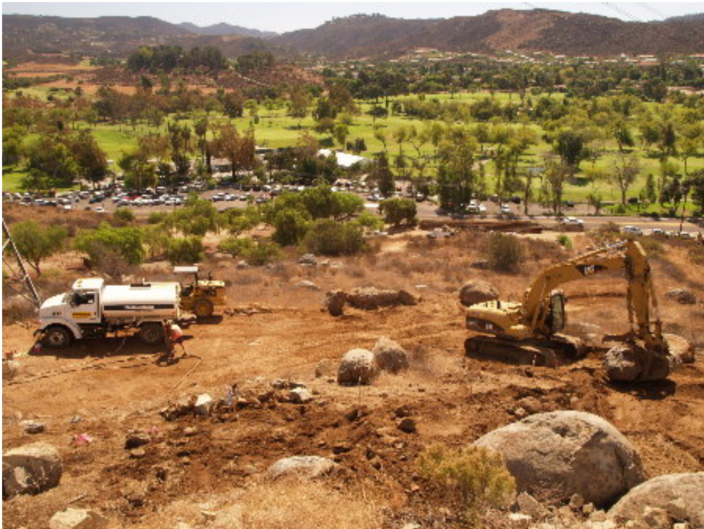
Figure 6 – The excavator operator at Tower Site 440 moved boulders off the pad for grading.
