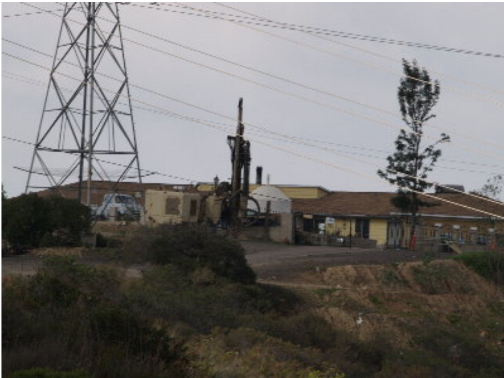
Figure 6 – The Air Track drilling machine moved to Tower Site 211, adjacent to a residence, to start work.
