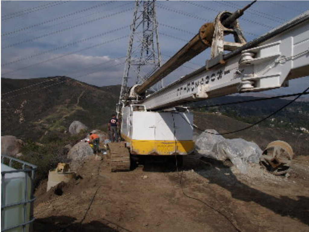
Figure 1 – The drilling machine at Tower Site 1300 was being repaired during the site visit.
