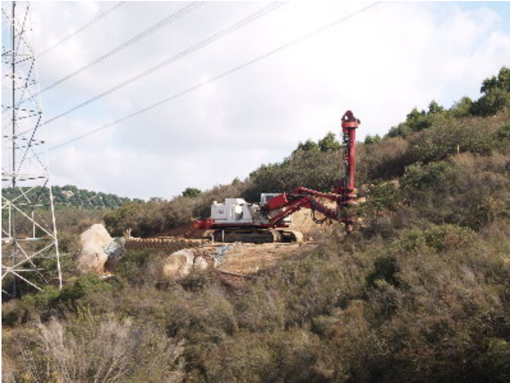
Figure 5 – The Low Drill at Tower Site 932 worked above the block wall on the pad site.
