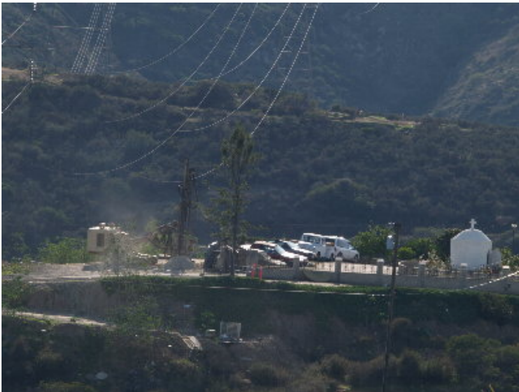
Figure 6 – The Air Track drilling machine continued at Tower Site 211, adjacent to a residence.
