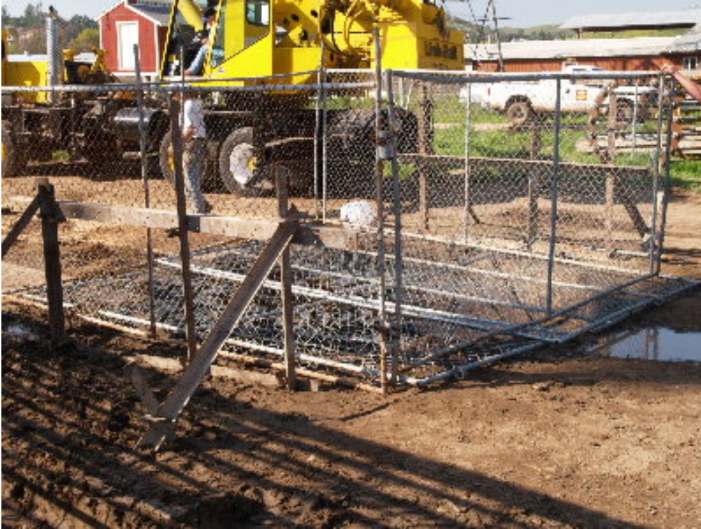
Figure 1 – Crews placed protective fencing over the completed foundation at Pole Site 1210 (the excavation failed overnight).
