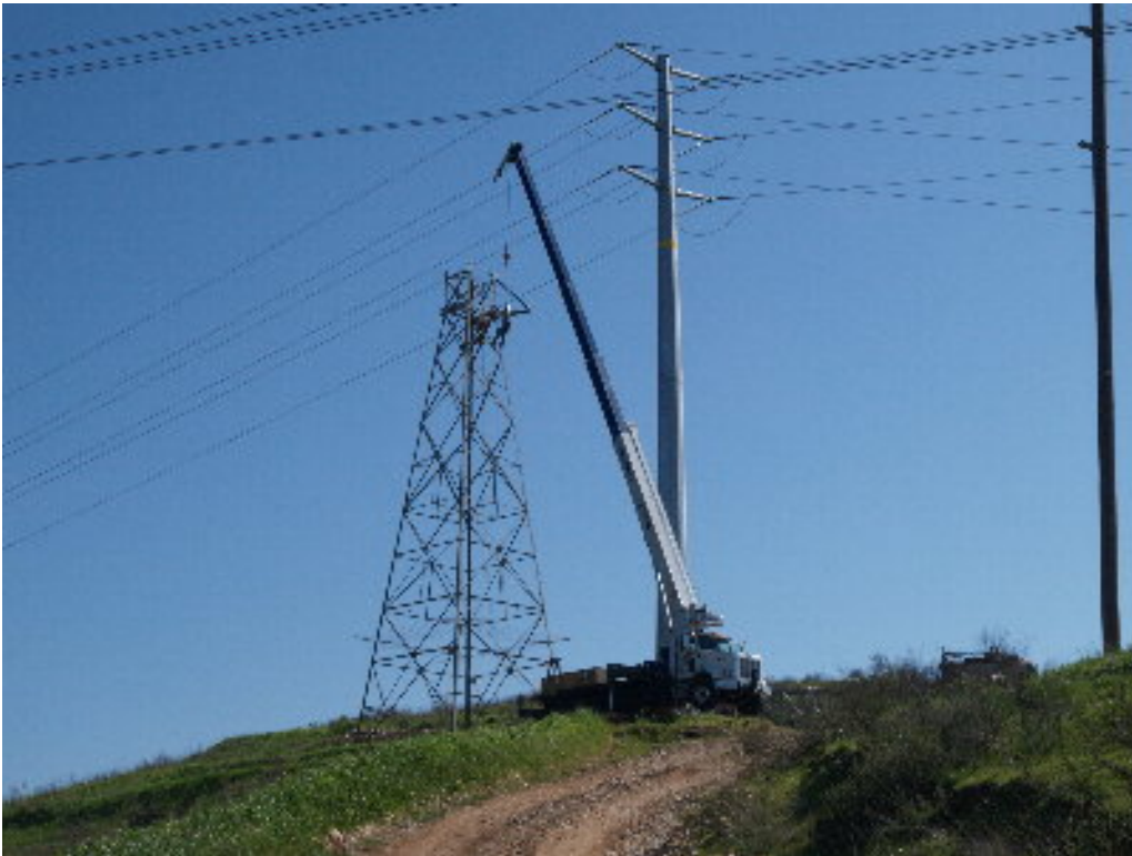
Figure 2 – The Wilson Construction crew worked to prepare the base for the modified upper section.
