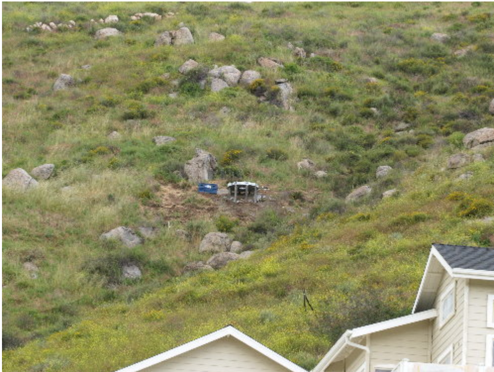
Figure 4 – The micro-pile crew work has been completed on the steep side-slope at Pole Site 493.
