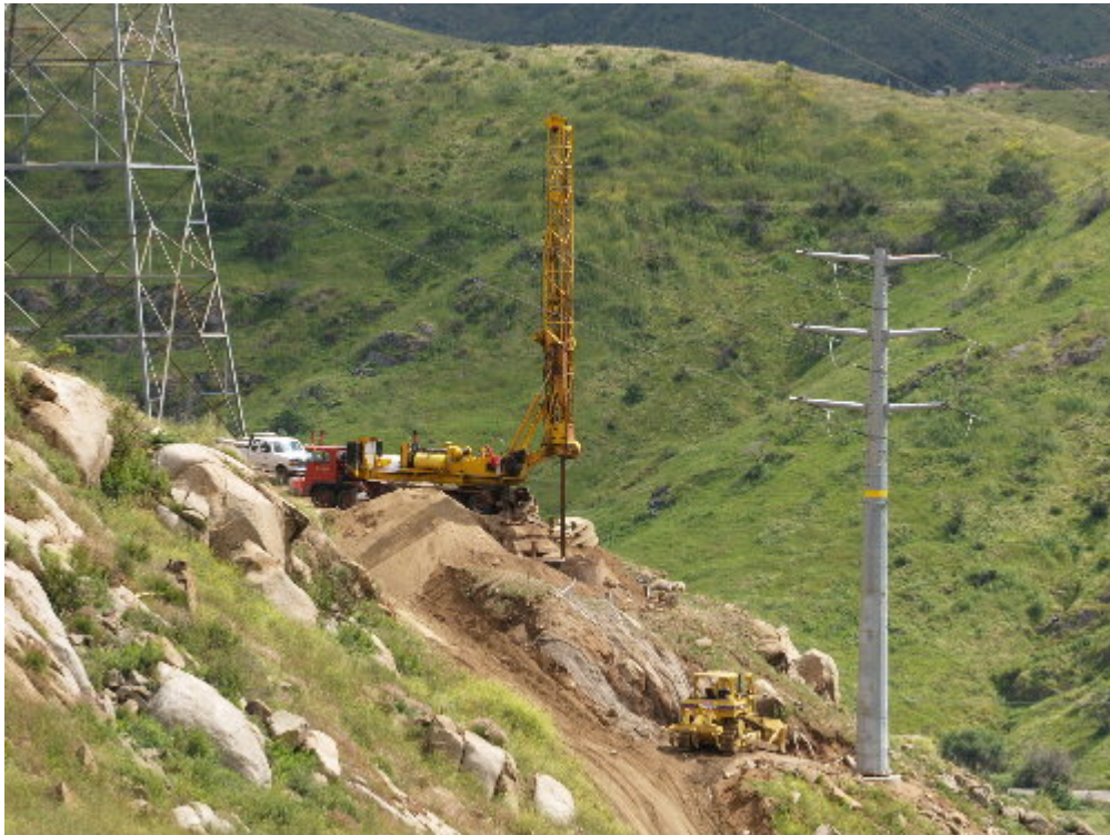
Figure 6 – Tri-State Drilling worked at Pole Site Z201915 to excavate the 230 kV foundation.
