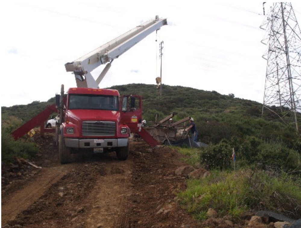
Figure 2 – PAR worked at Pole Site 172 to set the rebar cage and anchor bolts in preparation for pouring concrete.
