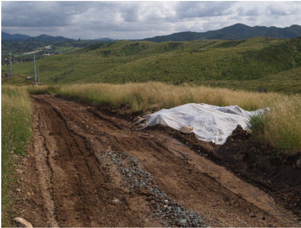
Figure 5 – The wet material pushed off the right-of-way at Fanita Junction has been covered and will be removed shortly.
