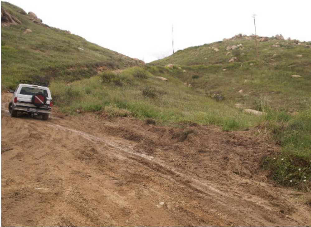
Figure 7 – An excavator traveled off the approved access road to Pole Site Z201914 and the area needs to be stabilized prior to any rains.
