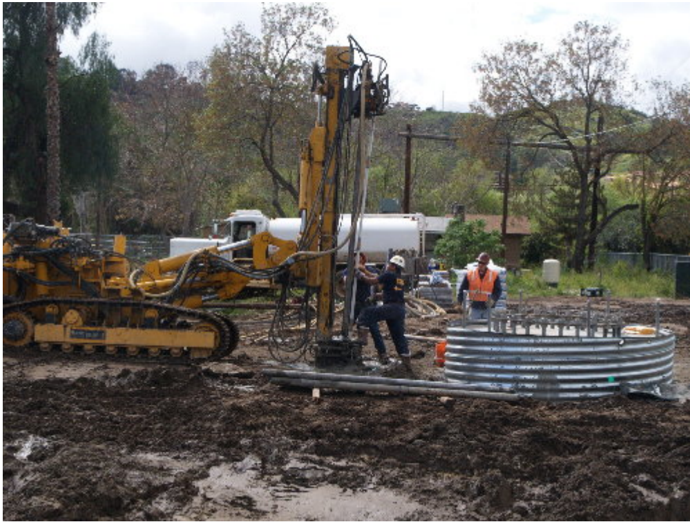
Figure 3 – The drilling and foundation pouring at Pole Site 1210 was completed on March 22 and crew prepared to pressure grout around the casing.
