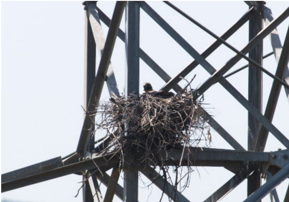
Figure 6 – An active red-tail hawk nest is just above the Los Coches Substation in a lattice tower.
