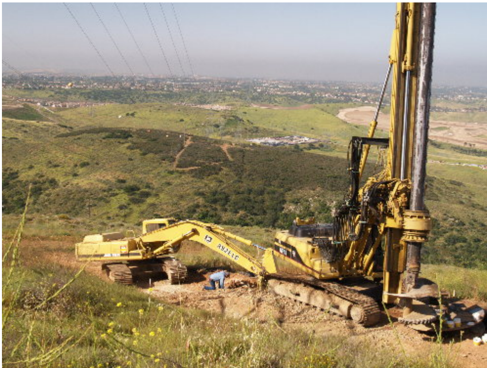
Figure 2 – The Woodward drilling crew worked at Pole Site 30 to complete the final 138 kV foundation excavation on the project.
