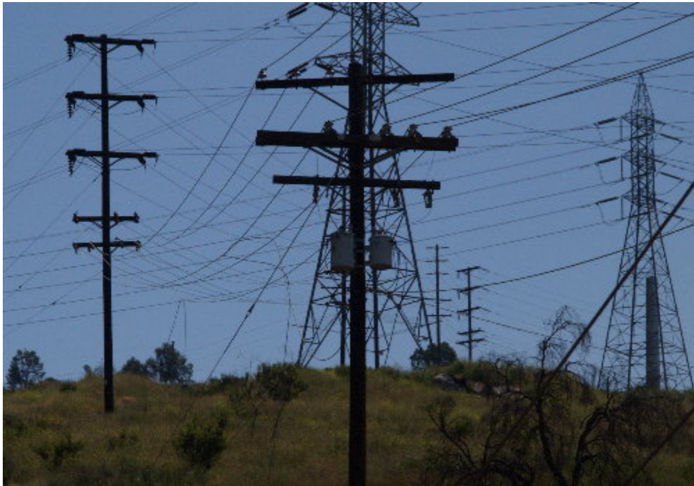
Figure 4 – A mobile crane struck a live 12 kV service line on the access road above the Los Coches Substation.
