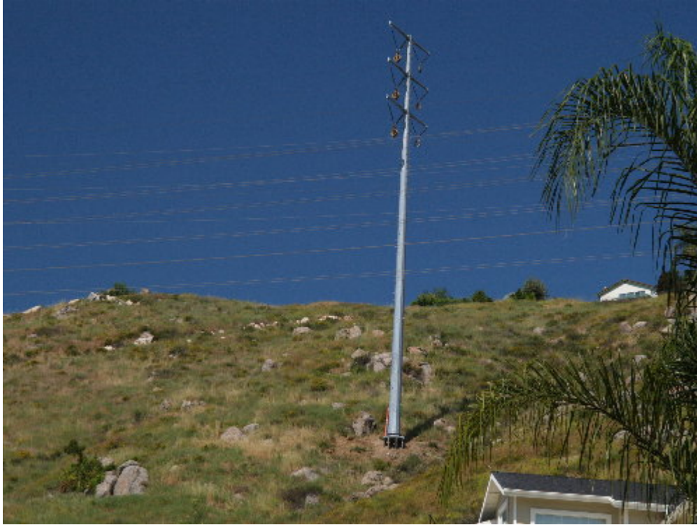
Figure 1 – A heavy-lift helicopter was used to set the steel pole sections at Pole Site 493.
