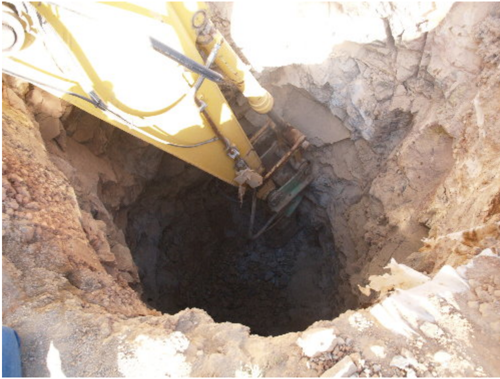
Figure 3 – The Woodward drilling crew at Pole Site 30 used a hydraulic hammer to break off the rock shelves on the sides of the excavation.
