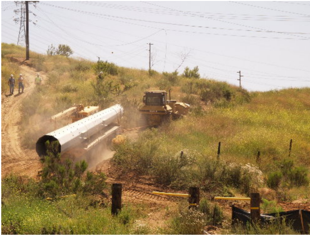
Figure 5 – Wilson moved the upper section of the steel pole up to the crane pad above Los Coches Substation.
