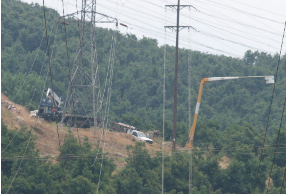
Figure 1 – The Wilson crew worked south of Interstate 8, preparing to lower the conductor with assistance of the helicopter.
