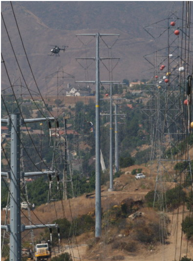
Figure 3 – Wilson used a helicopter to hold the conductor off the avocado trees.
