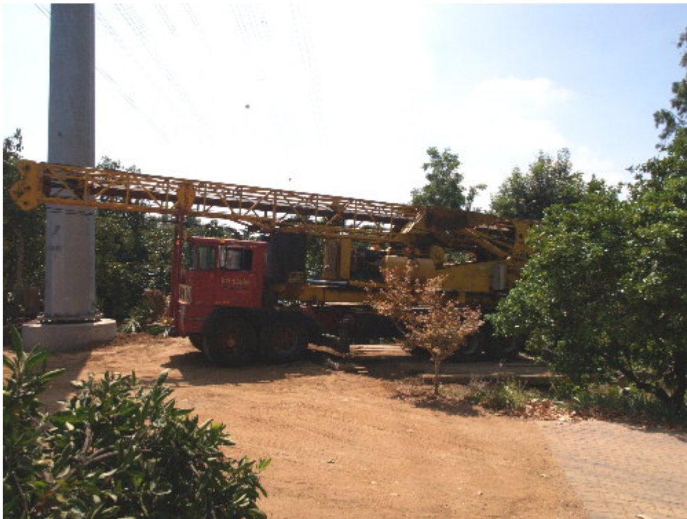
Figure 3 – The Tri-State drilling crew set up the drilling machine at Singing Vista.
