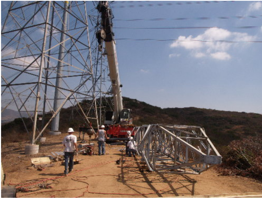
Figure 4 – The Wilson tower modification crew worked above Steele Canyon High School during the site visit.
