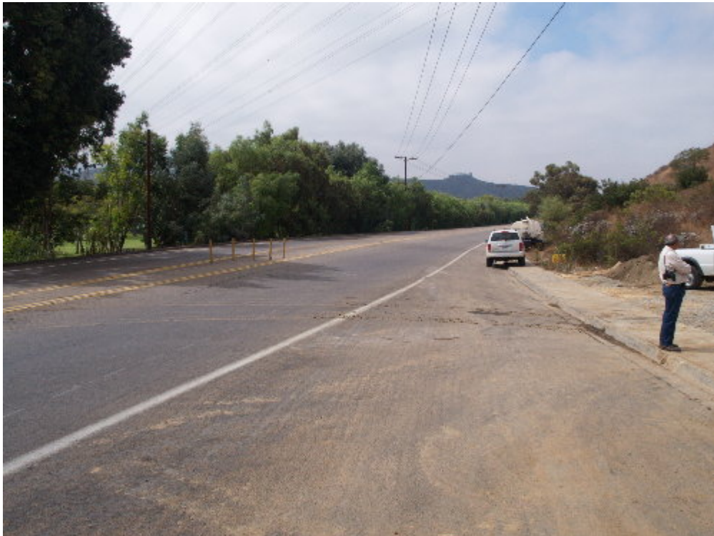
Figure 5 – All material tracked onto the public right-of-way is cleaned up at the end of each shift.
