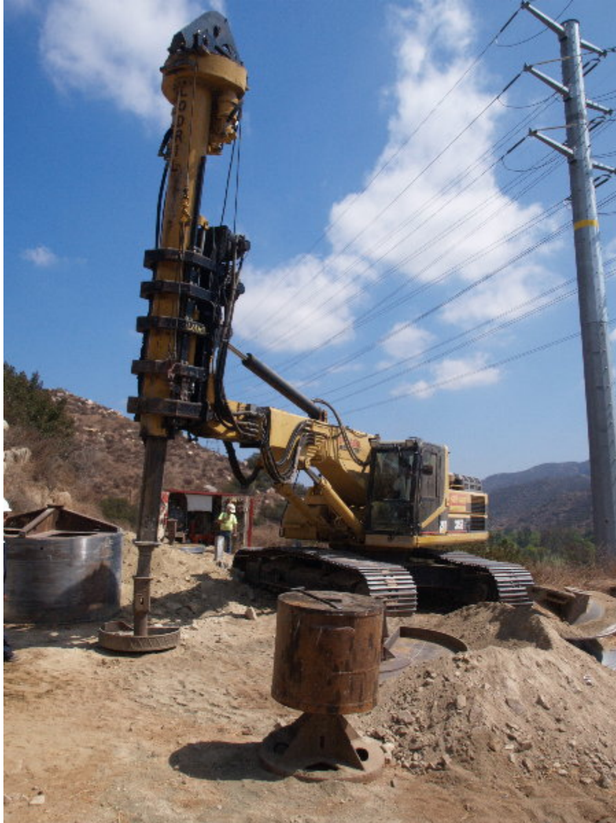
Figure 1 – The Tri-State drilling completed the excavation on the turning pole foundation above Willow Glen.
