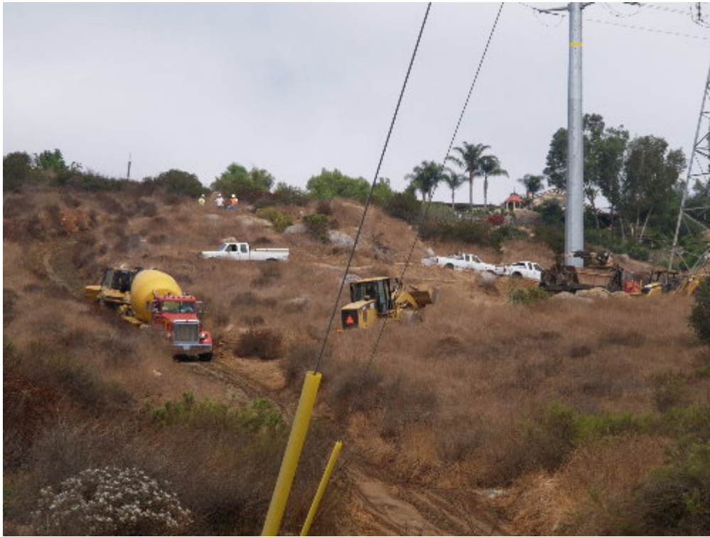
Figure 2 – The concrete trucks were pulled up the steep slope by the bulldozer.
