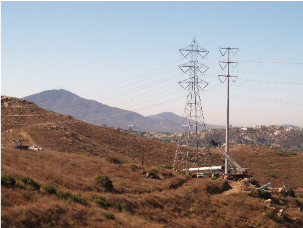
Figure 2 – Wilson unloaded steel pole sections at Camino Monte Sombra in preparation to raise the pole.
