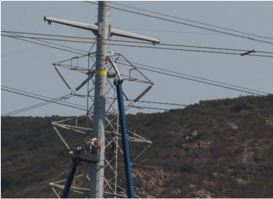
Figure 3 – A Wilson crew worked to secure the tower sections above the Miguel Substation.
