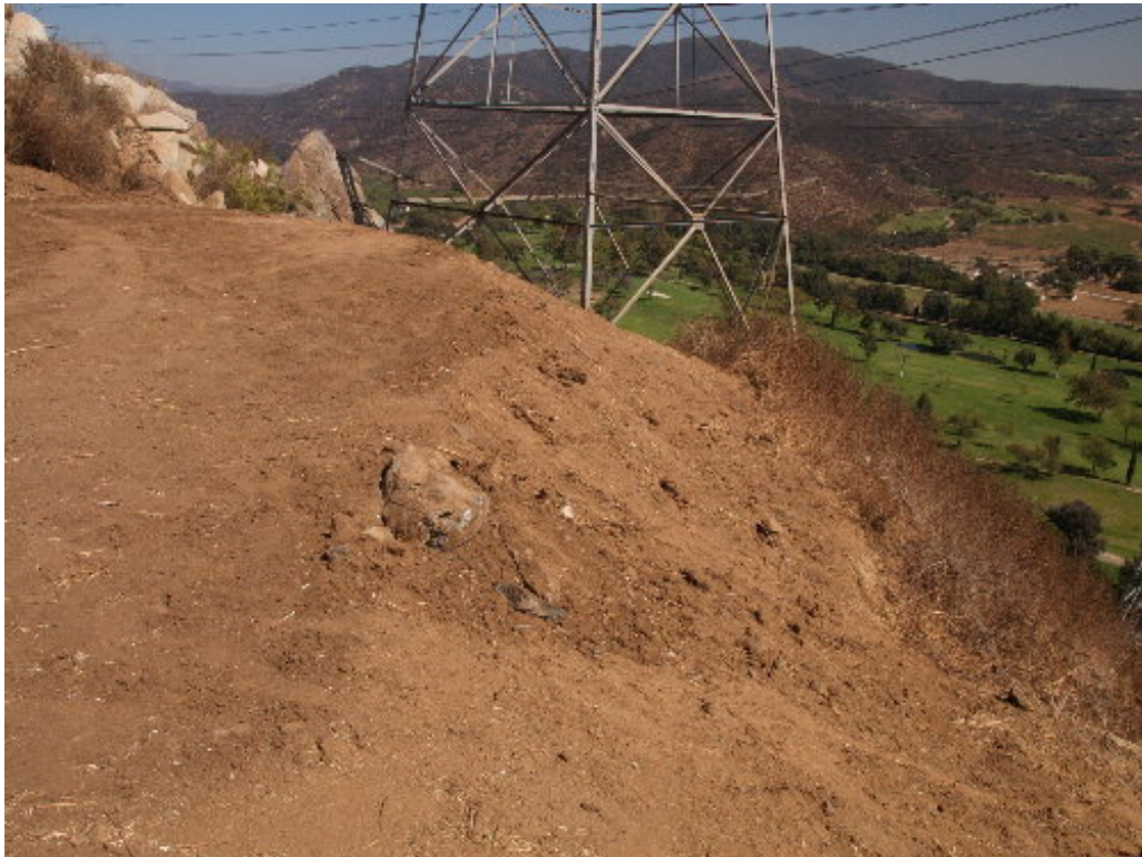
Figure 4 – The pad used by Wilson during the tower modification below Wind River Road needs to be stabilized prior to any rainfall.
