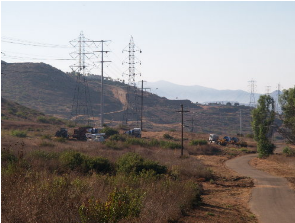
Figure 2 – The reel trucks were staged in the approved stringing site east of La Cresta while crews waited for the right-of-way to dry.
