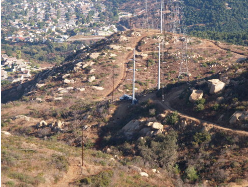
Figure 1 – Boom trucks were staged at modified towers and new steel pole sites in preparation for the stringing activities.
