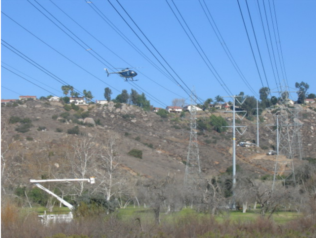
Figure 1 – A helicopter was used to install the rope for tower stringing on Wednesday, January 18 th across the Cottonwood Golf Course.
