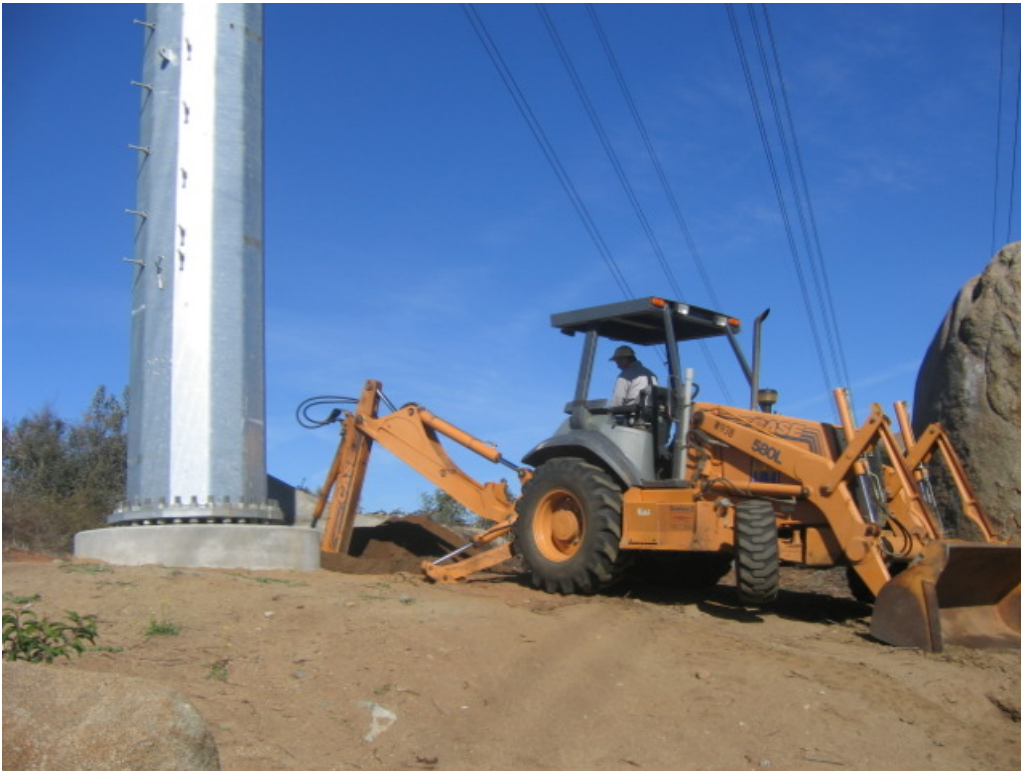
Figure 2 – Wilson crews used a backhoe to install the grounding system for the new steel poles.
