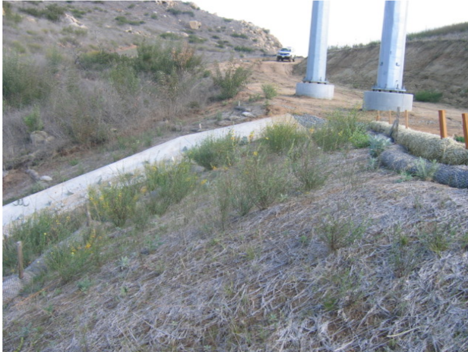
Figure 1 – Restoration area from last year along Camino Monte Sombre. This area has been netted and re-growth is apparent.
