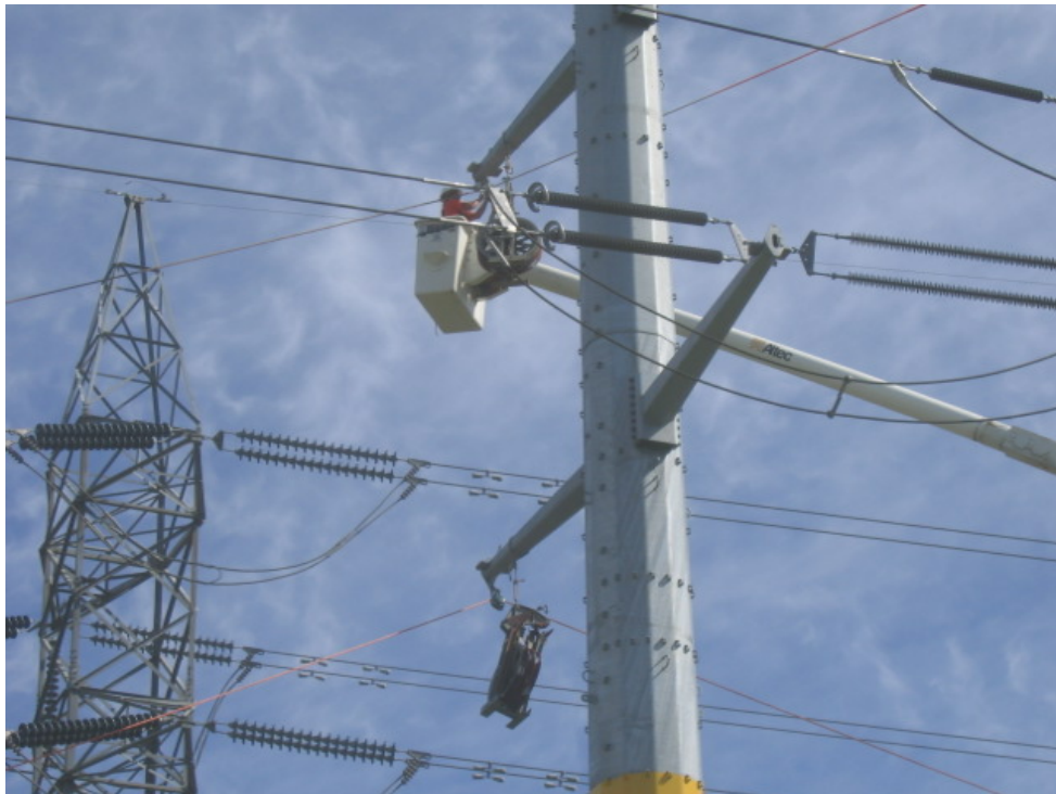
Figure 2 – PAR crews completed the last section of wire installation in the Fanita to Los Coches segment.
