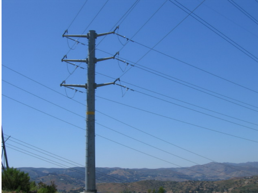
Figure 1 – Sturgeon crews working on the temporary 230 kV lines near Lake Jennings. Conductor was moved from an existing steel lattice tower and replaced onto a new steel pole.
