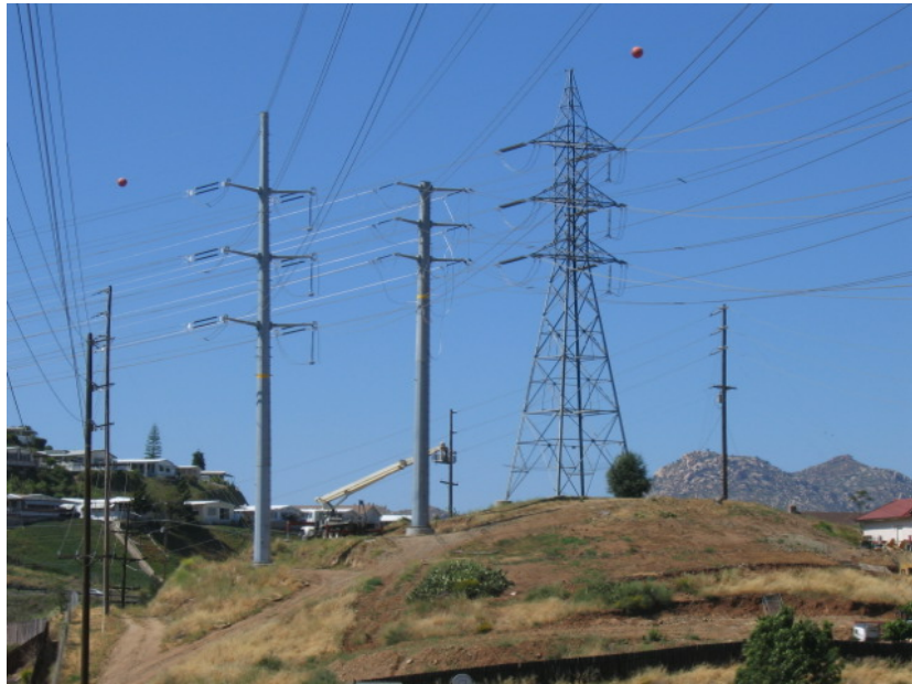
Figure 2 – Guard structures and an abandoned lattice tower were removed after the put back was completed.
