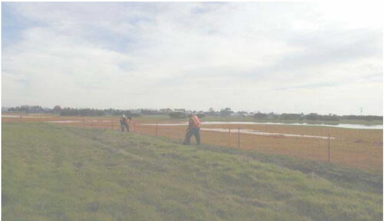
Figure 3 Crew Digging a Trench for Silt Fence Installation at Catella Property January 3, 2003
