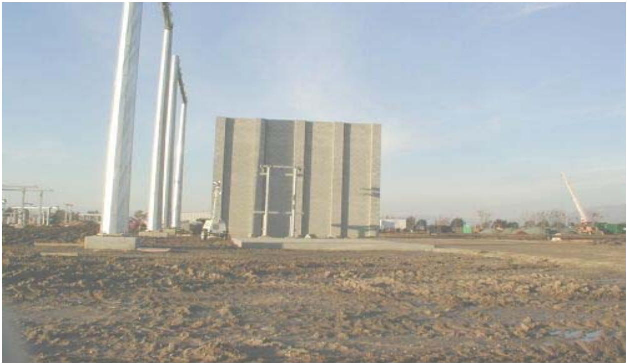
Figure 5 Fire Wall and Transformer Pad at the Los Esteros Substation January 3, 2003
