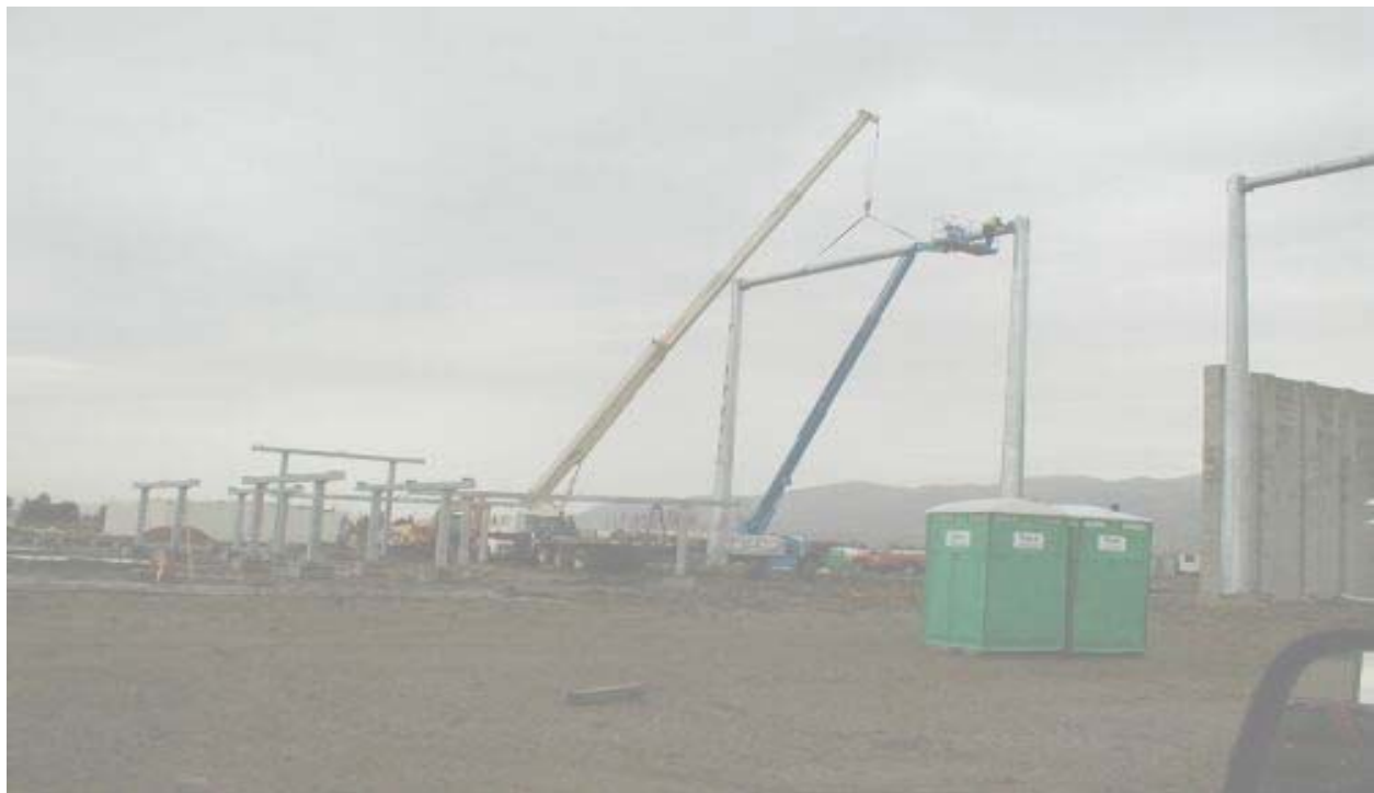
Figure 1 Crews Using Crane to Erect Steel Poles at the Los Esteros Substation December 30, 2002
