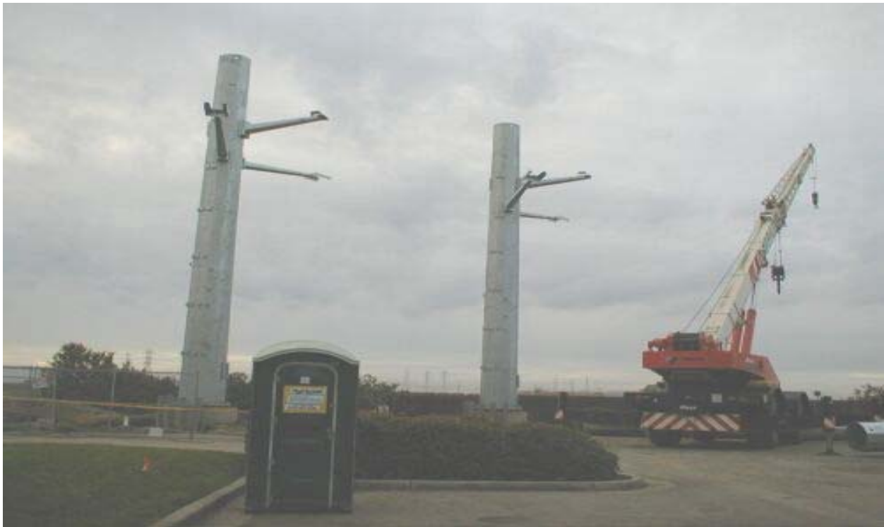
Figure 3 Poles 9(a) and (b) being Erected at West End of Cushing Parkway January 24, 2003
