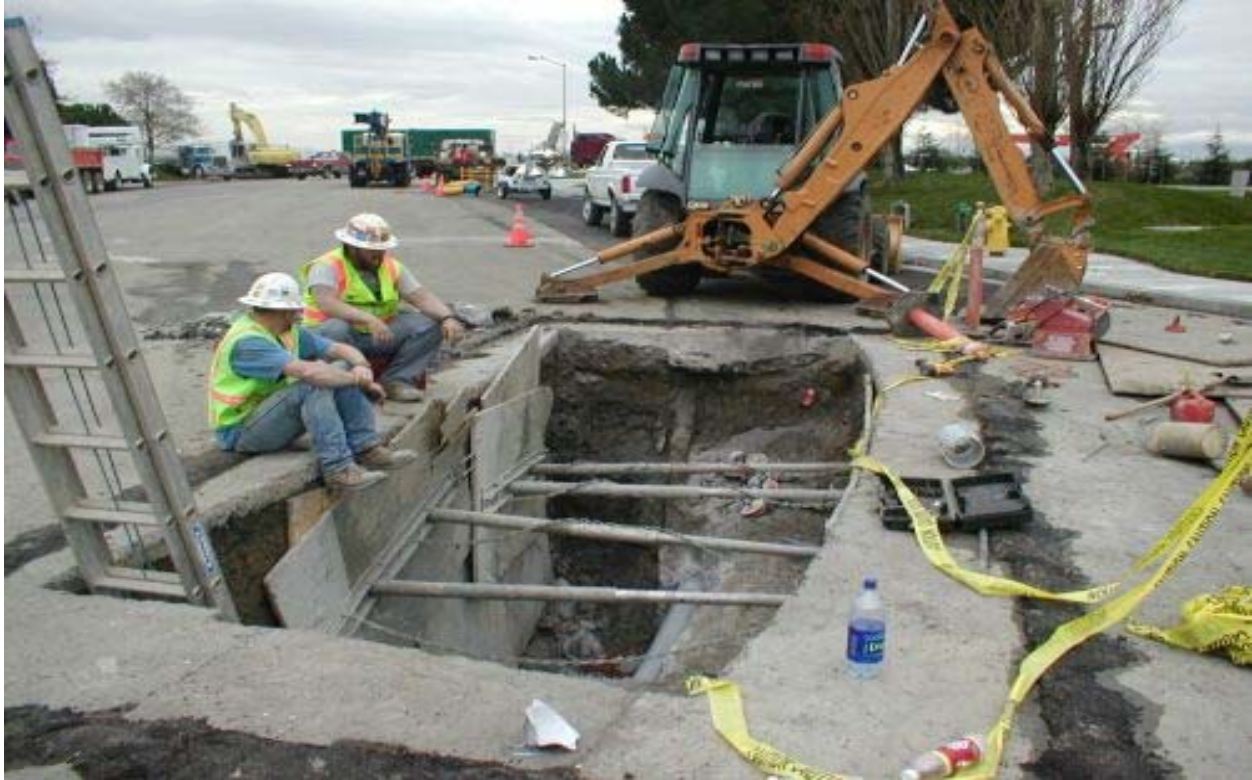
Figure 2 Proofing Problems on Right Line Trench North of Man-hole Vault #10 January 21, 2003
