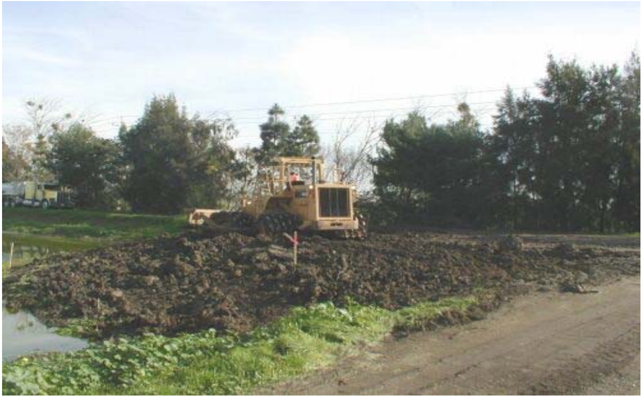
Figure 4 Crew Creating Pad for Pole Foundation #25 at San Jose Water Treatment Plant January 24, 2003
