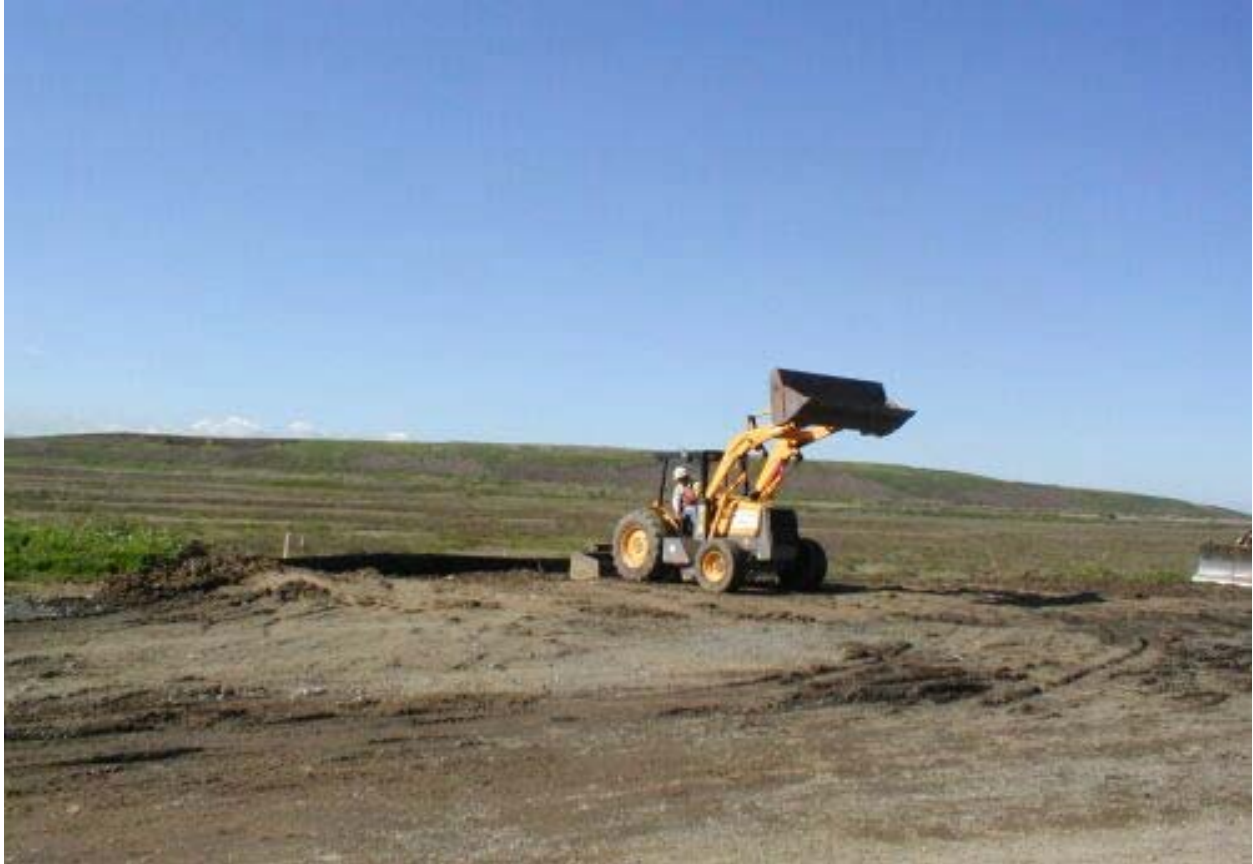
Figure 3 Appian Crews Creating Pole Foundation Pad at Pole area #12(a) and (b) on the King & Lyon's Property February 18, 2003
