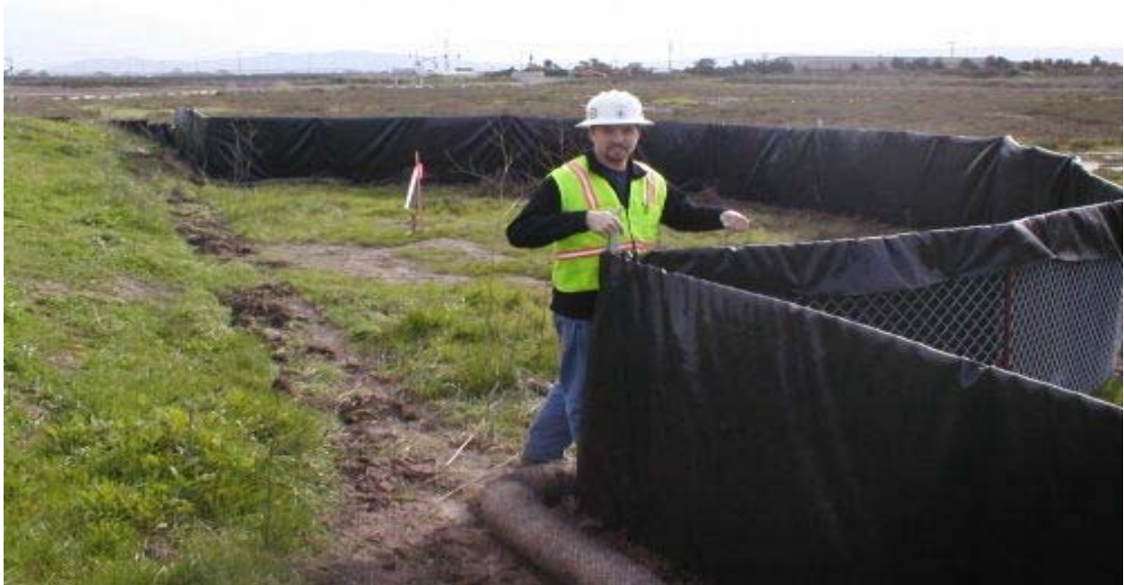
Figure 1 Silt Fence around Pole Area #12(a) and (b) on the King & Lyon's Property February 17, 2003
