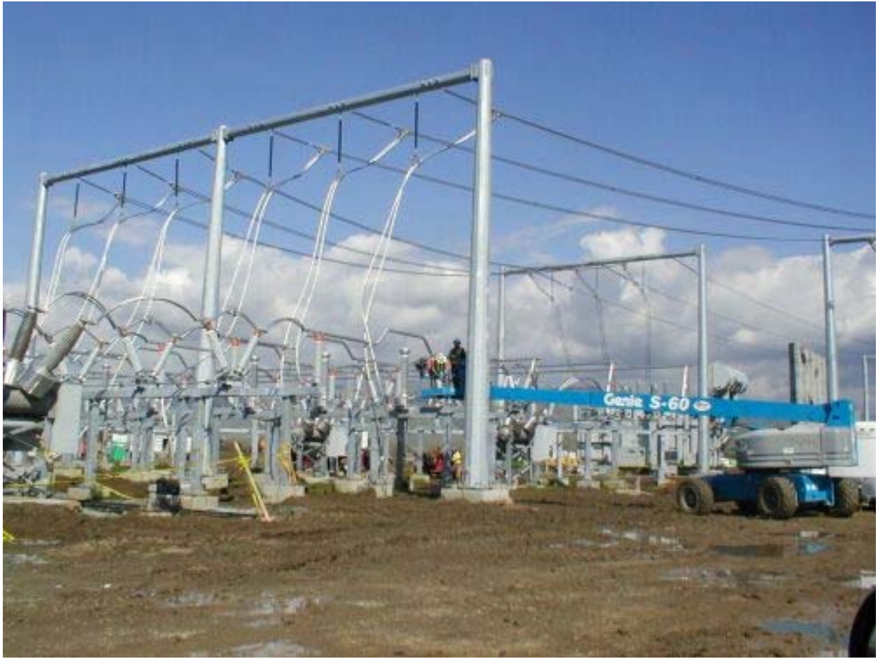
Figure 3 Los Esteros Substation February 27, 2003
