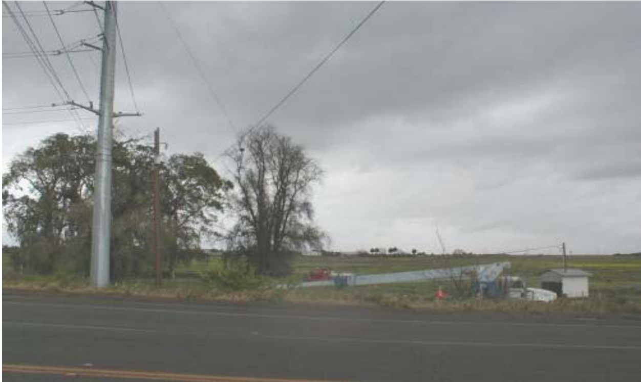
Figure 1 OPGW Stringing on West Side of Zanker Road Near Red-tailed Hawk's Nest April 12, 2003
