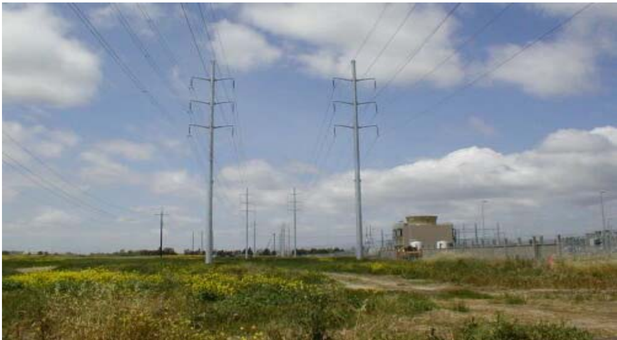
Figure 2 Pole Towers in Field West of Los Esteros Substation May 7, 2003
