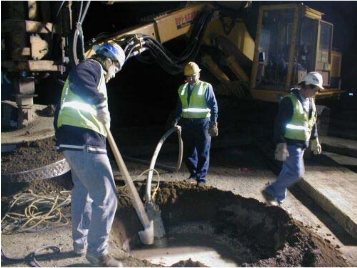
Figure 3 Trimble – Montague Segment Crews Dewatering Pole Foundation Pit #10 Where Water Line Broke May 15, 2003
