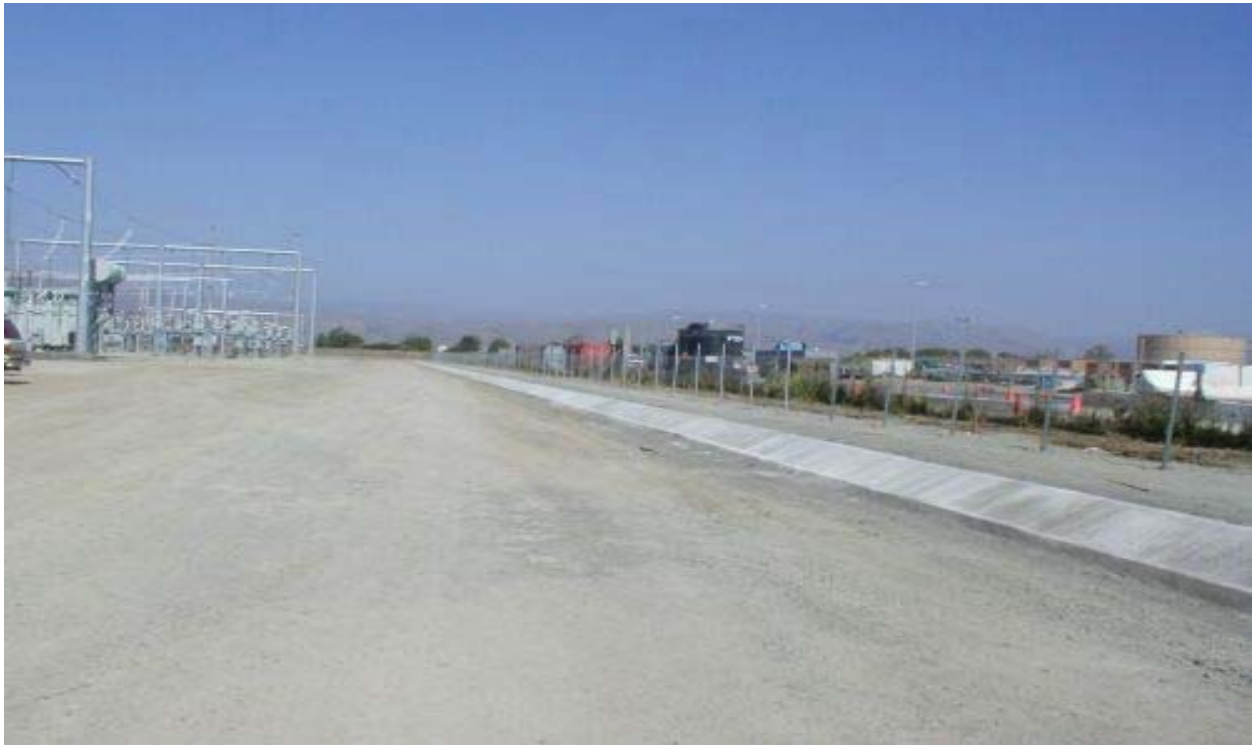
Figure 2 New Drainage Ditch on East Side of Los Esteros Substation Site May 15, 2003
