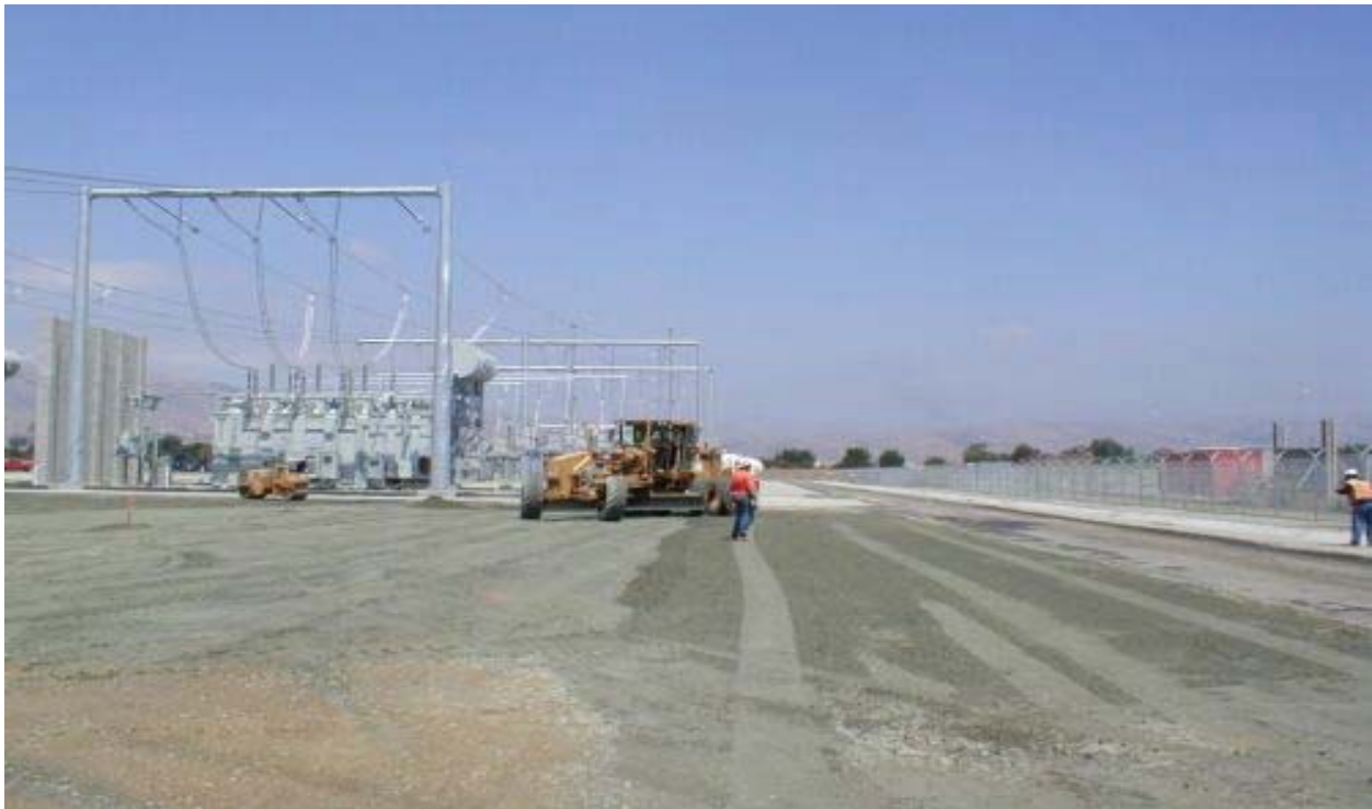
Figure 2 Appian Crews Laying and Compacting Base Rock at the Los Esteros Substation May 30, 2003
