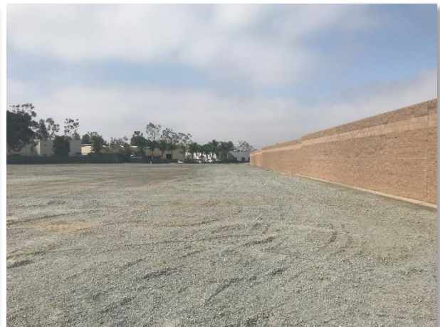
Figure 7. Class 2 base rock and perimeter block wall was installed around the future substation site
