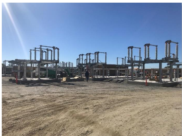
Figure 10. Steel and insulator installation on foundations at the Ocean Ranch Substation, January 23, 2019
