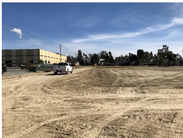
Figure 4. AM Ortega crews conducted grading and soil export activities at the Ocean Ranch Substation site
