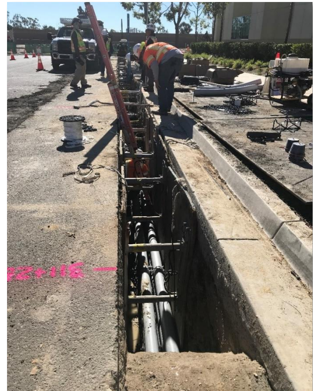
Figure 17. Trenching on Rocky Point Drive was followed by conduit installation and concrete backfill, January 23, 2019
