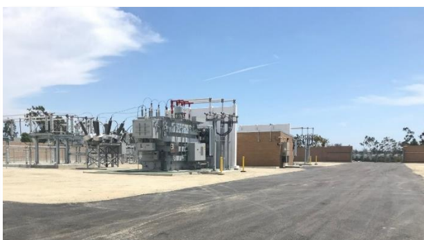
Figure 13. Crews completed final paving of the interior access road within the Ocean Ranch Substation, July 23, 2019
