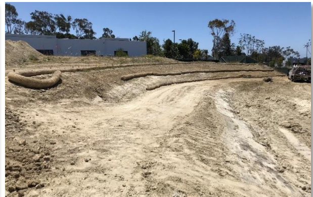
Figure 23. BMPs (straw wattles) were installed along slopes for sediment control which are inspected and maintained regularly
