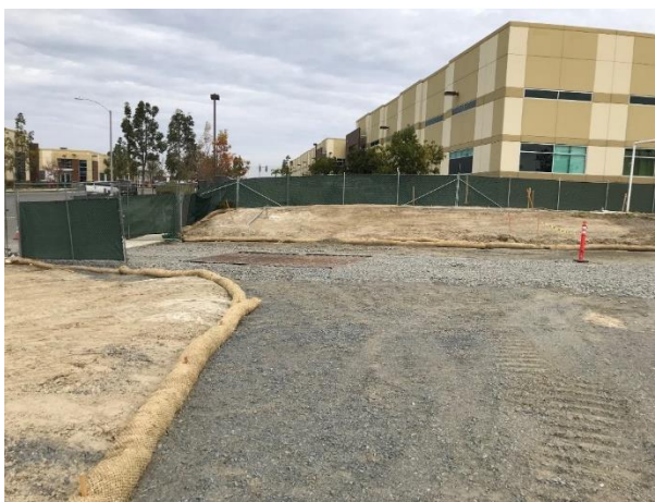
Figure 5. New driveway with sediment controls installed at the Ocean Ranch Substation site
