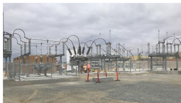
Figure 12. Chain link fencing surrounding the substation components has been completed at the new, low-profile Ocean Ranch Substation, May 7, 2019
