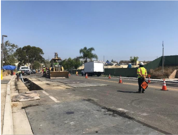
Figure 14. Trenching and conduit installation for the Loop in work being conducted along Avenida Del Oro, July 25, 2018
