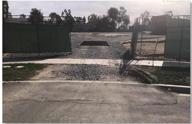
Figure 25. Stabilized construction entrance was observed to be in need of maintenance, December 4, 2018
