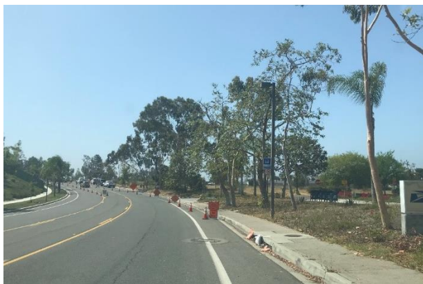
Figure 20. Traffic controls are in place and lanes are open during construction on Avenida Del Oro
