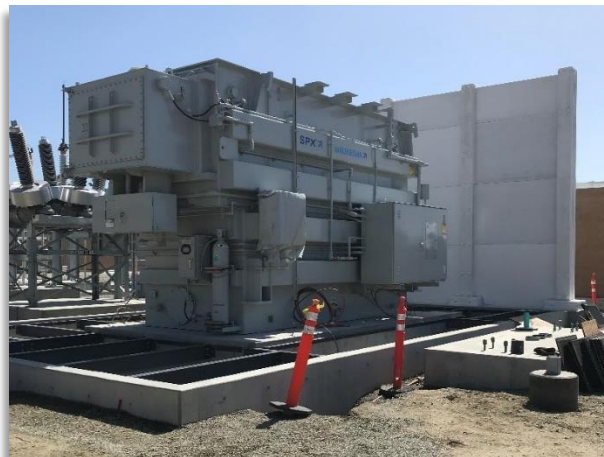
Figure 11. Transformer delivery and installation along with newly constructed fire walls inside the substation, March 13, 2019
