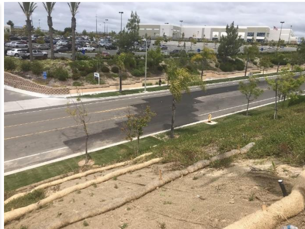
Figure 19. BMPs were installed and new landscaping was planted along slope disturbed by 12 kV trenching work between the Ocean Ranch Substation and Avenida Del Oro, May 7, 2019
