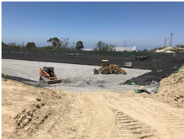
Figure 6. Once the basin liners were installed, sand and gravel were brought in for drainage
