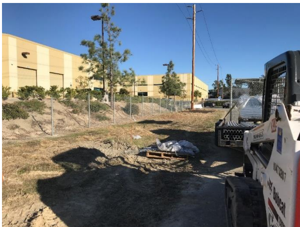
Figure 3. Chain link perimeter fencing was installed at the Ocean Ranch Substation site
