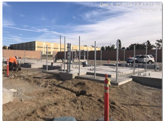
Figure 9. Steel and fence post assembly on newly constructed foundations at the Ocean Ranch Substation, December 4, 2018
