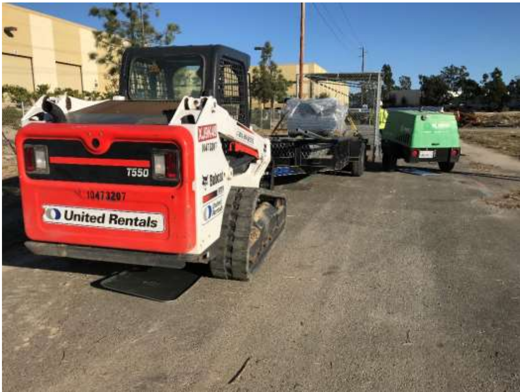
Figure 3 – Equipment staged at the Ocean Ranch site with dip pans placed underneath.
