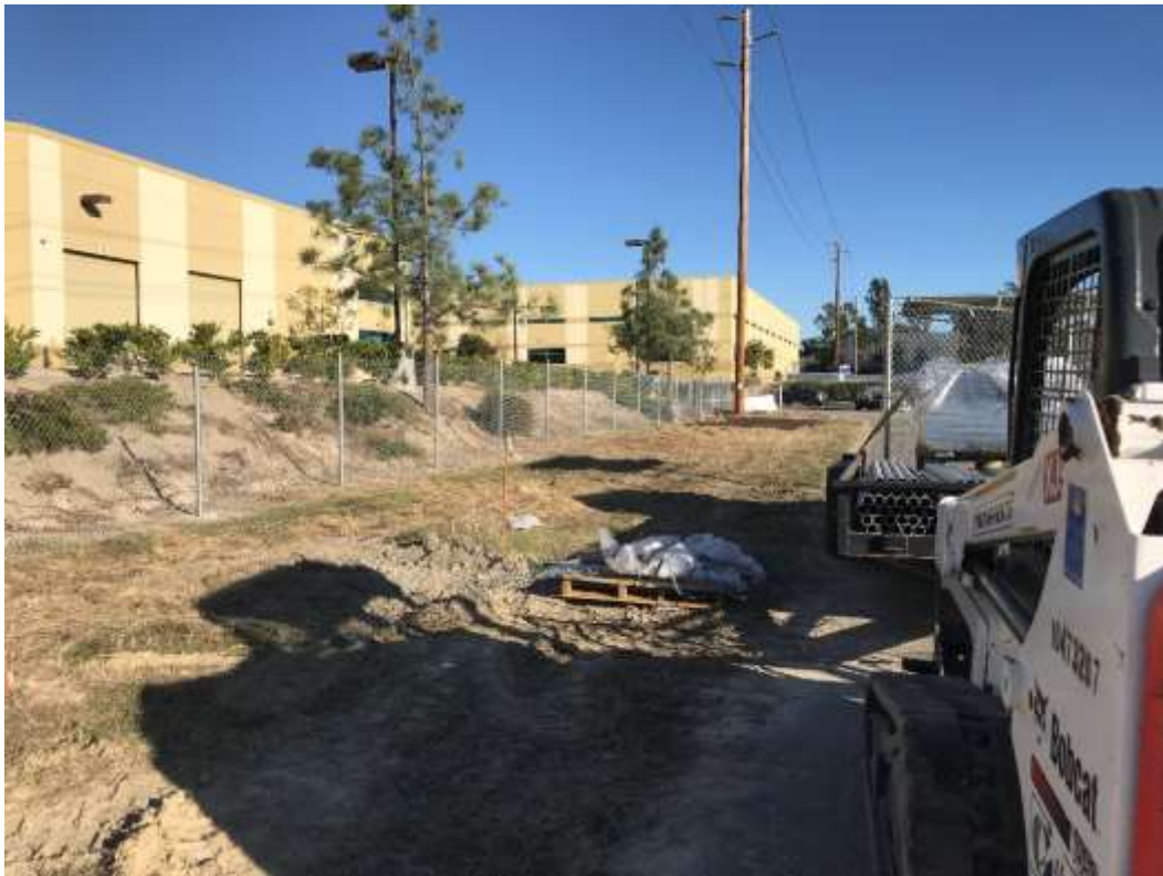
Figure 2 – Chain link perimeter fencing was installed at the Ocean Ranch Substation site.
