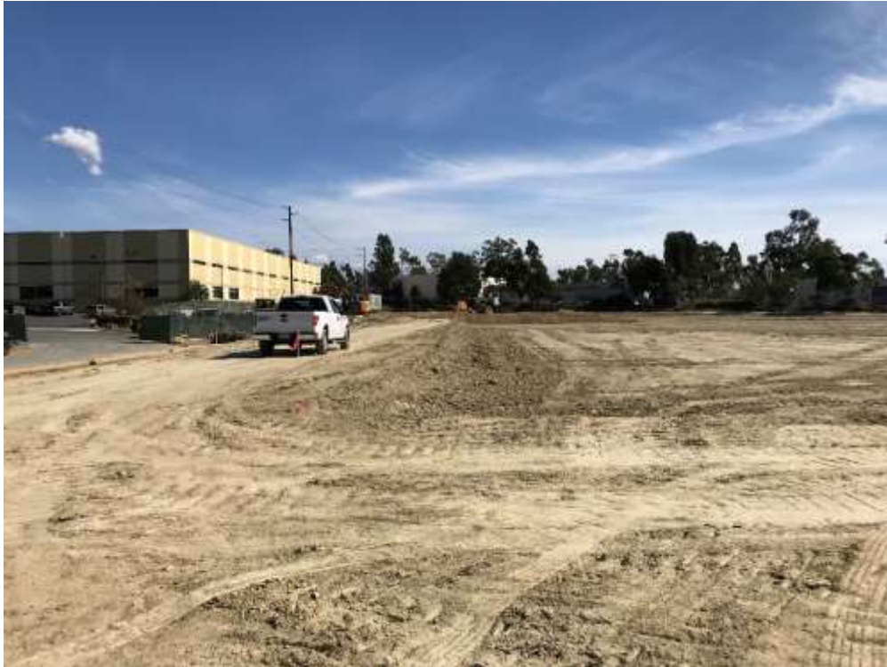
Figure 1 – AM Ortega crews conducted grading and soil export activities at the Ocean Ranch Substation site.
