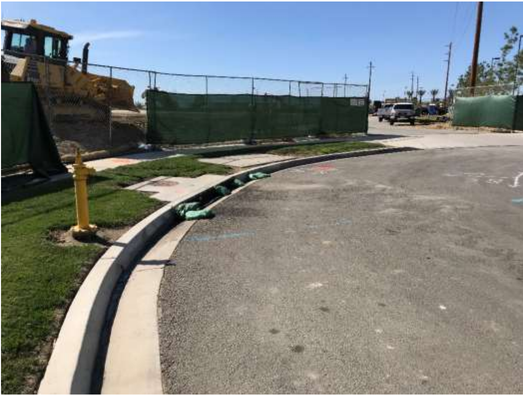
Figure 3 – BMPs, including inlet protection, were installed near the Substation entrance.
