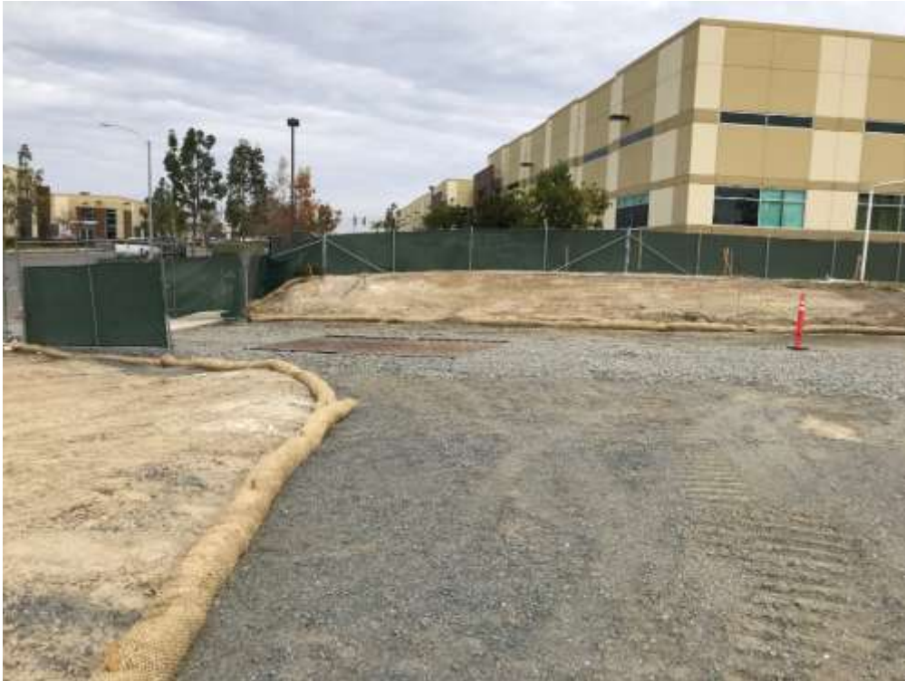
Figure 1 – New driveway with sediment controls installed at the Ocean Ranch Substation site.
