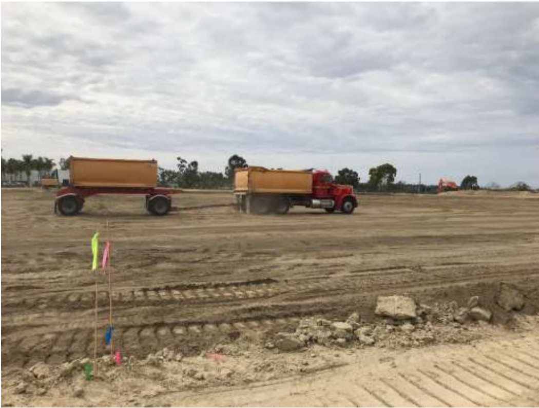
Figure 3 – Soil import continues at the Substation entrance. Trucks are limited to using the stabilized entrance when exiting the site.
