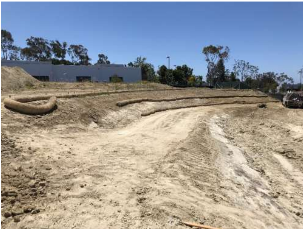
Figure 2 – BMPs (straw wattles) were installed along slopes for sediment control which are inspected and maintained regularly.
