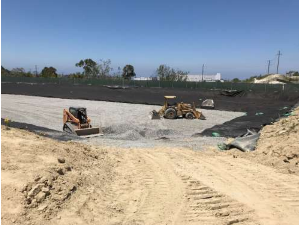
Figure 1 – Once the basin liners were installed, sand and gravel were brought in for drainage.
