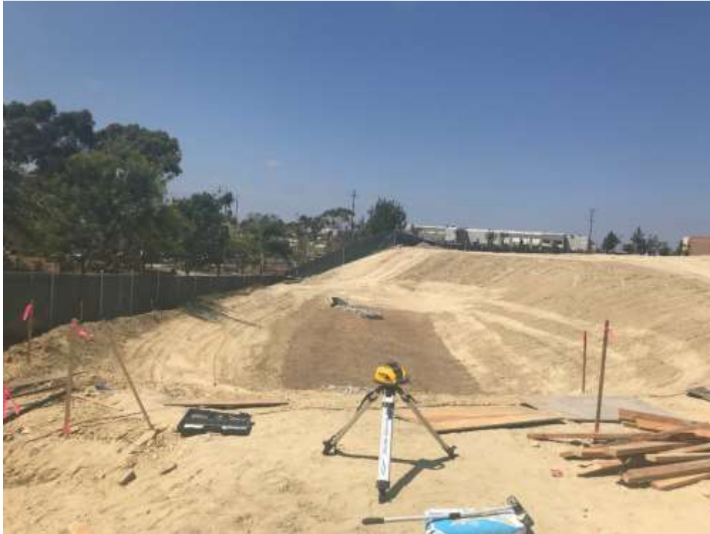
Figure 1 – Installation of rock and sand for filtration was completed at the southwest drainage basin, August 15, 2018.
