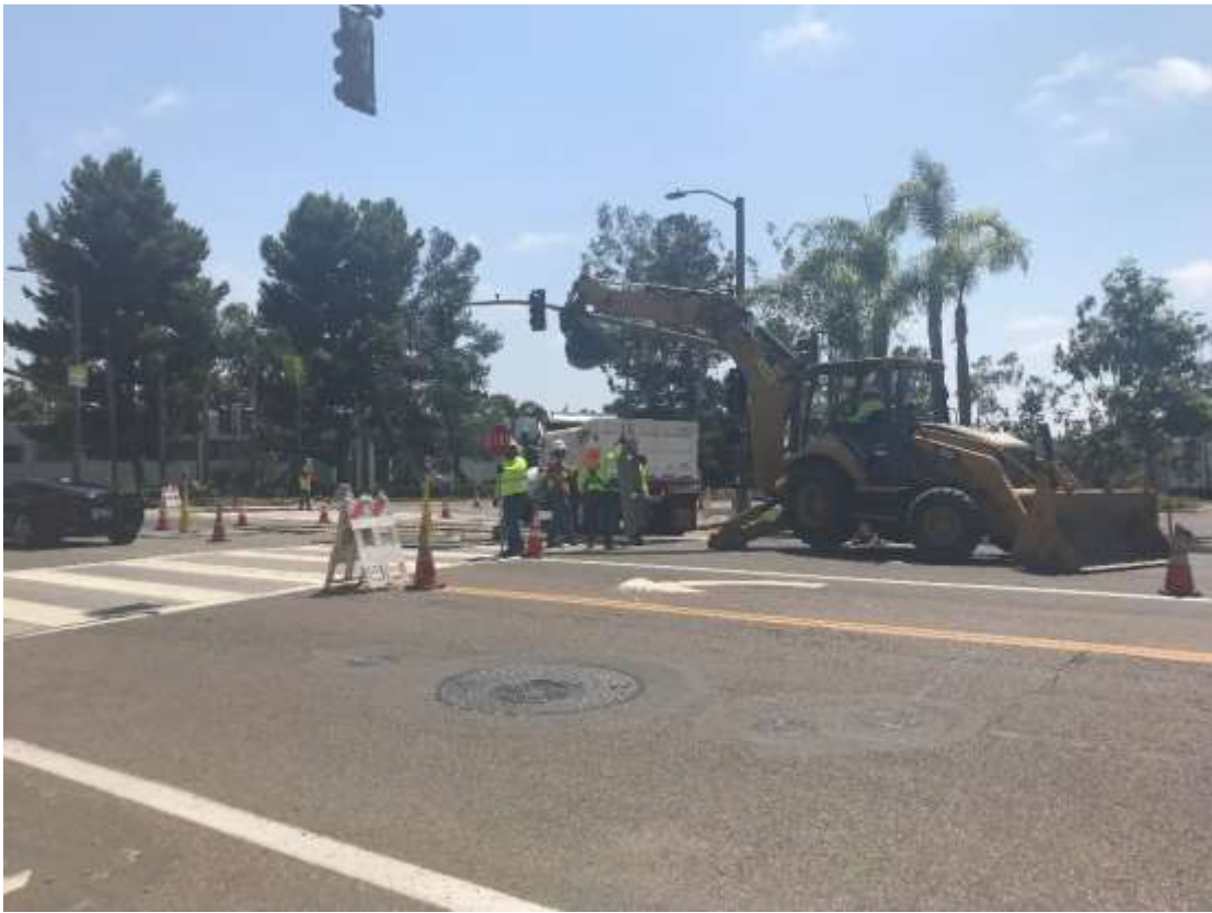
Figure 3 – Trenching and conduit installation for the Loop In work being conducted along Avenida Del Oro and Avenida De La Plata, August 15, 2018.
