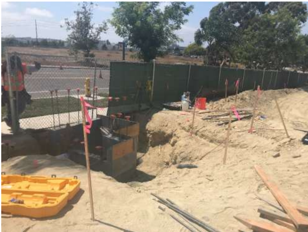
Figure 2 – Concrete forms were built as part of the basin drainage system on site, August 15, 2018.
