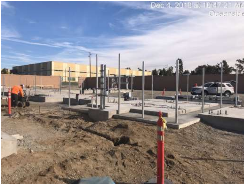
Figure 1 – Steel and fence post assembly on newly constructed foundations at the Ocean Ranch Substation, December 4, 2018.
