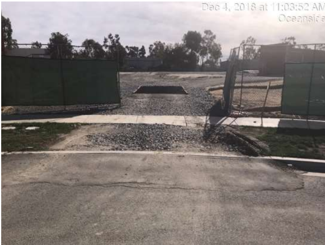
Figure 3 – Stabilized construction entrance was observed to be in need of maintenance, December 4, 2018.
