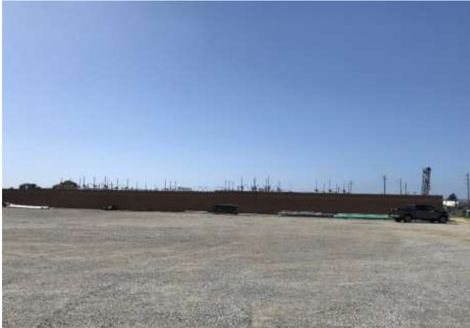
Figure 1 – Steel and insulator installation continues at the new, low-profile Ocean Ranch Substation, March 13, 2019.
