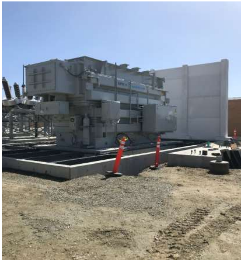
Figure 2 – Transformer delivery and installation along with newly constructed fire walls inside the substation, March 13, 2019.
