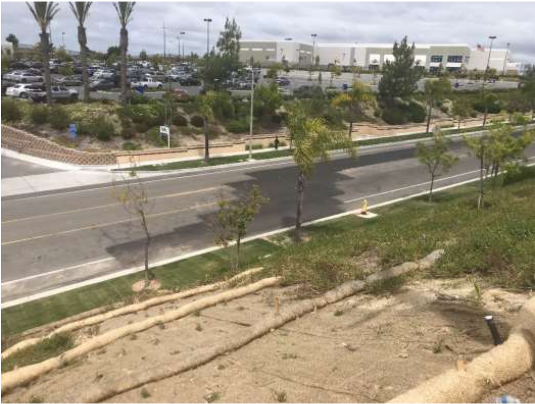
Figure 3 – BMPs were installed and new landscaping was planted along slope disturbed by 12 kV trenching work between the Ocean Ranch Substation and Avenida Del Oro, May 7, 2019.
