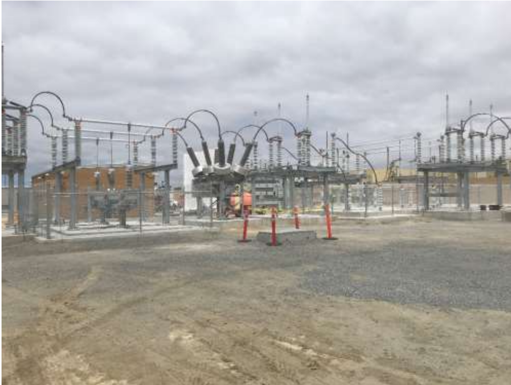
Figure 1 – Chain link fencing surrounding the substation components has been completed at the new, low-profile Ocean Ranch Substation, May 7, 2019.
