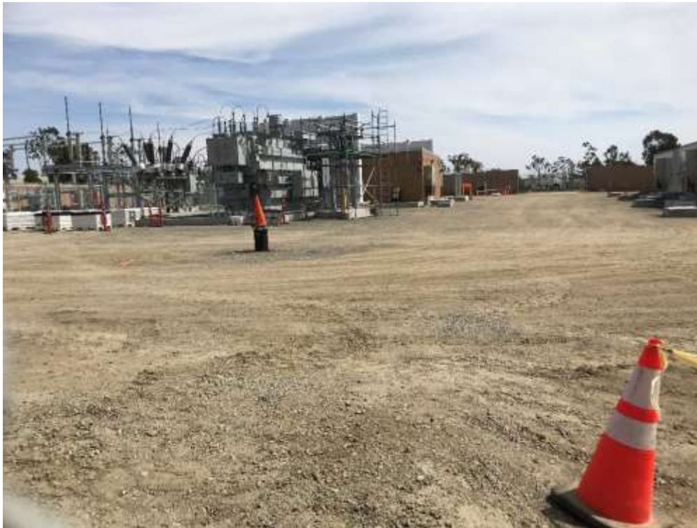
Figure 1 – Crews continued with control shelter wiring and overhead component installation at the new, low-profile Ocean Ranch Substation, June 11, 2019.
