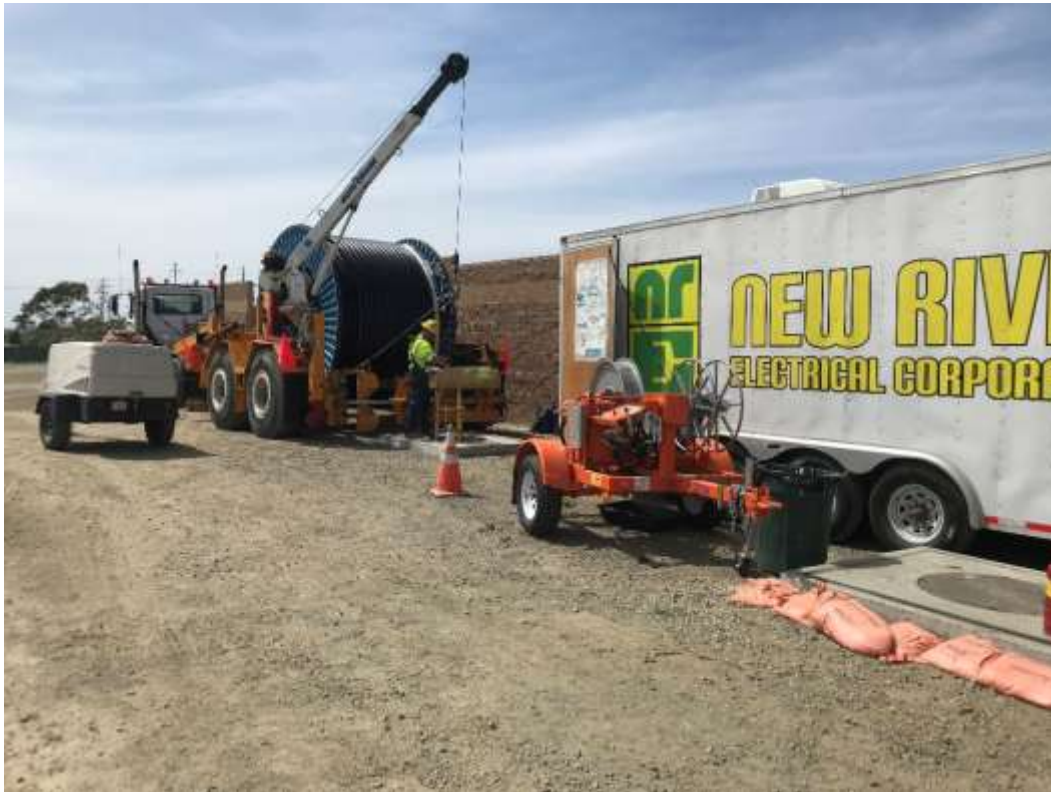
Figure 3 – New River Electric pulling 69 kV electric cable through underground vaults outside of the substation, June 11, 2019.
