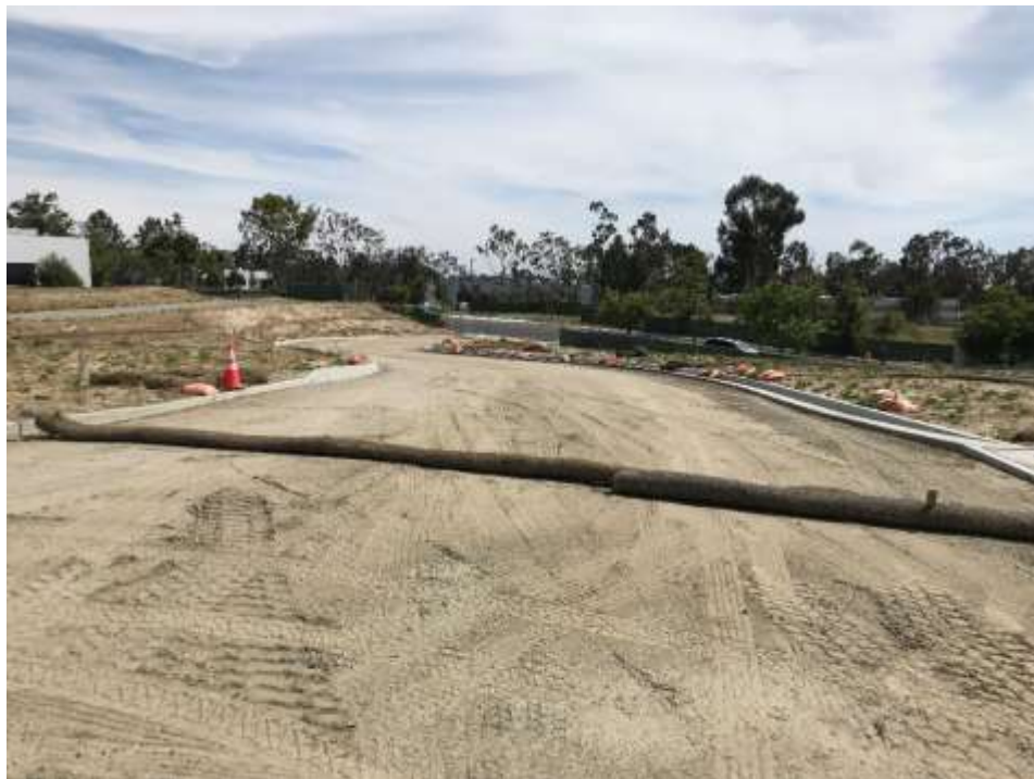
Figure 2 – Class 2 base is being distributed along the new driveway and adjacent access roads, June 11, 2019.
