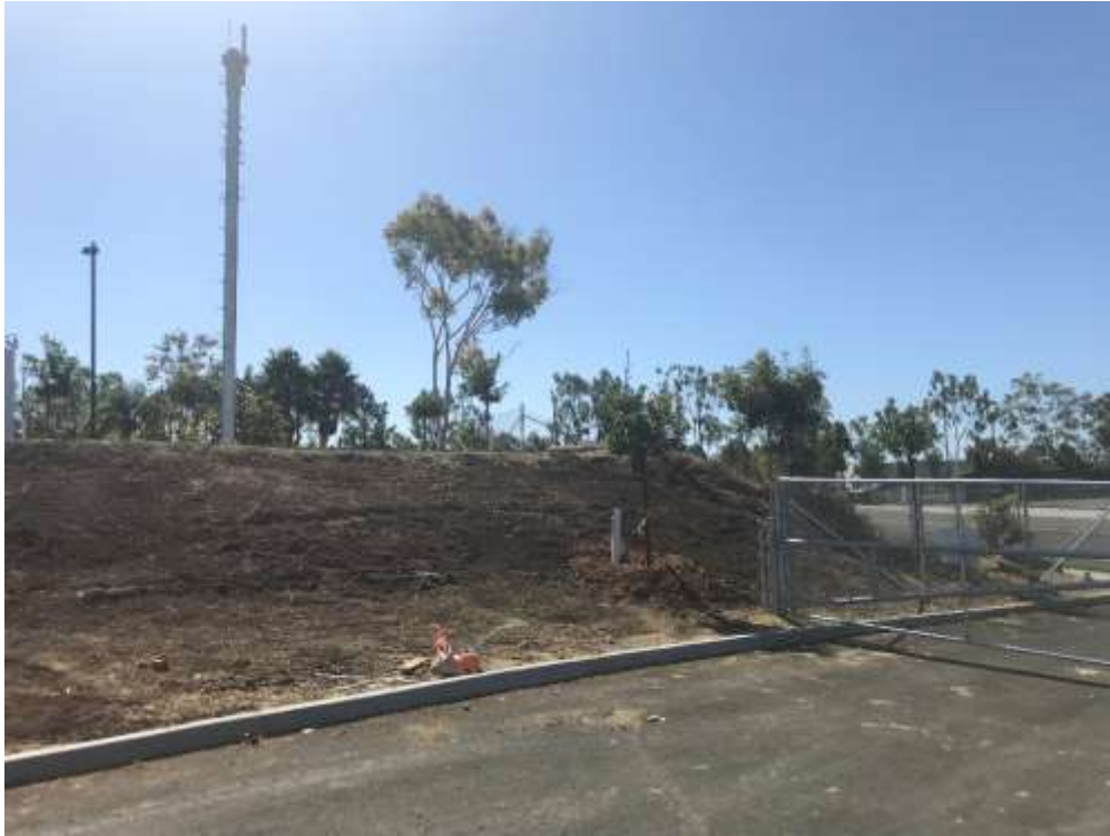
Figure 3 – The monopole was set at the south corner of the Project boundary, October 4, 2019.
