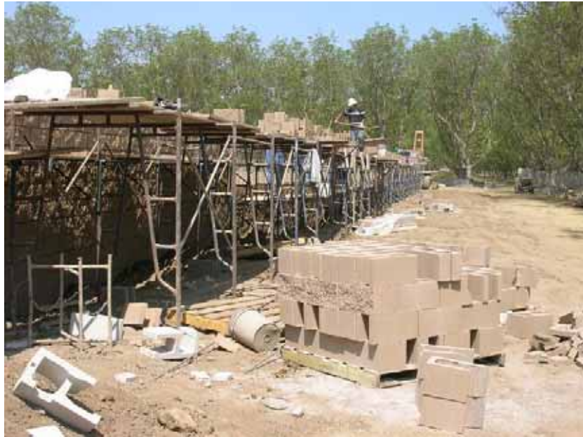
Figure 1: The substation perimeter wall construction was underway. The wall has been designed to match nearby new housing tract perimeter wall appearance. The photograph is of the east side of the wall, and faces northward.
