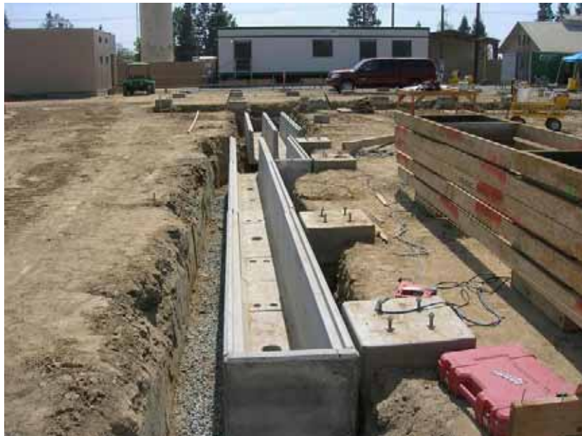
Figure 4: There were several trenches two feet and greater deep. These trenches were provided with wood ramps at the close of each work day in order to prevent trapping of wildlife. The temporary SCE construction trailer can be seen in the middle background. The MEER room is on the left. The building in the distant right corner is off site. The photograph faces southward.
