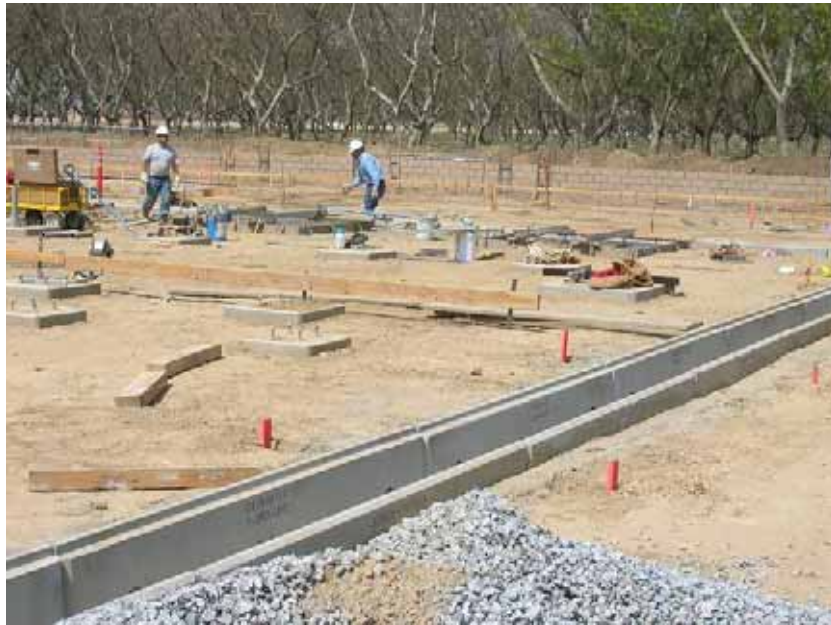
Figure 3: The construction of the underground power grid construction was underway. The photograph faces northwestward.
