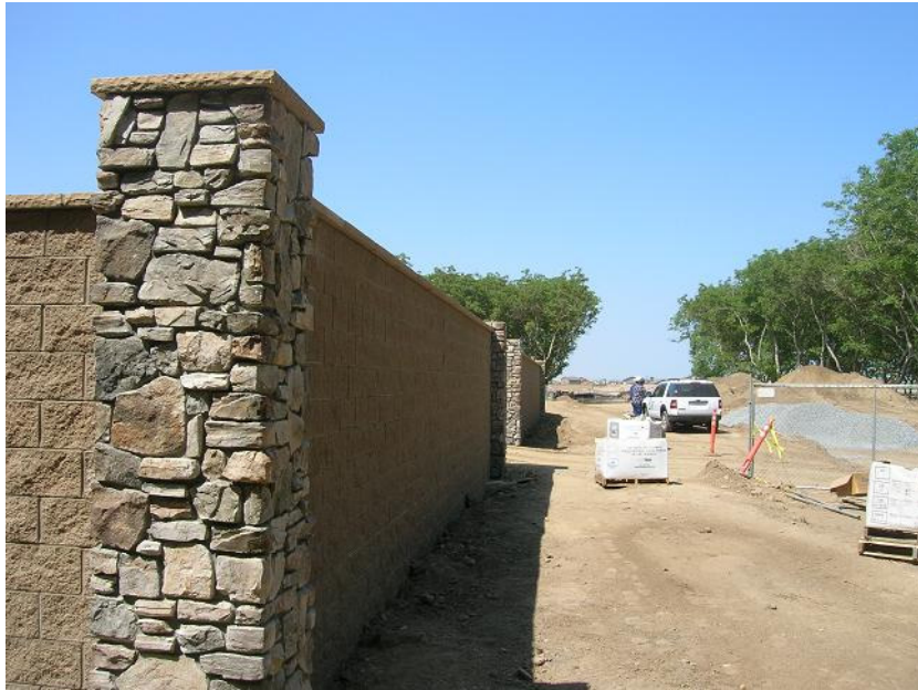
Figure 1: The perimeter wall was mostly completed. The design of the wall, including pillars and capstones, is intentionally similar to nearby housing tracts. The photograph faces westward along the route of the future permanent entrance road.
