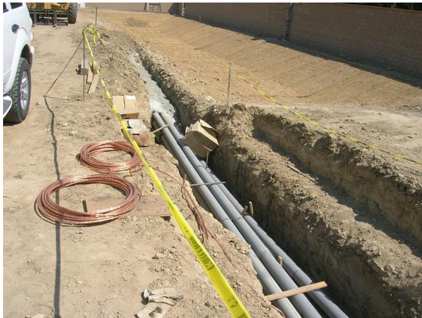
Figure 3: Conduit construction included trenching, placement of conduit, and grouting over the placed conduit.
