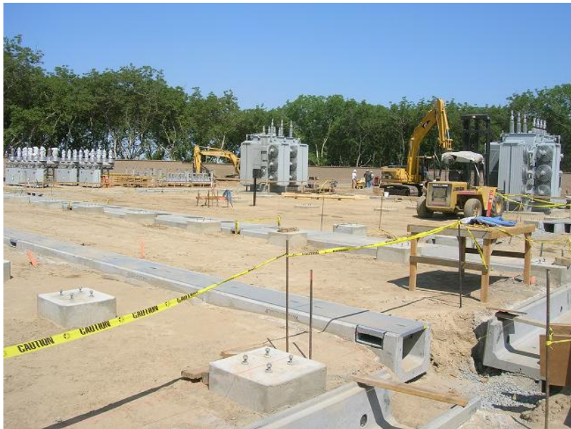
Figure 2: Civil work continued, including installation of concrete pads, concrete footings, and conduit. The photograph faces northwestward.
