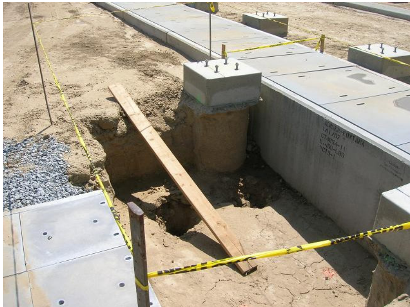
Figure 4: Wildlife ramps continued to be placed in all trenches two or more feet deep.
