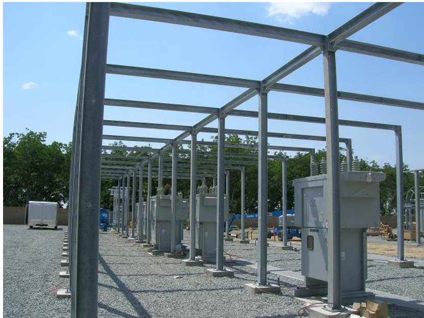
Figure 4: Installation of the transformers, capacitor banks, and circuit breakers continued. The photograph faces westward.
