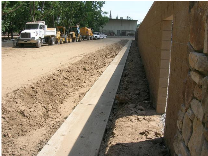
Figure 3: The incoming drain on the outside of the east perimeter wall for the retention basin was still under construction. The photograph faces southward.
