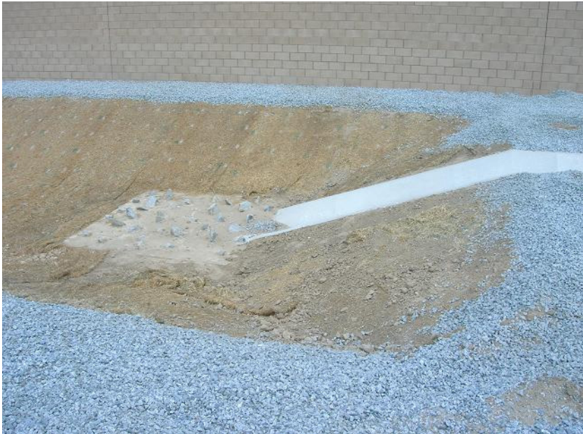
Figure 1: The water runoff retention basin was almost completed. The water force dissipation structure was in place.
