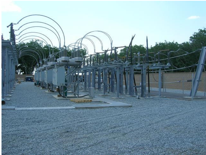
Figure 5: Installation of the transformers, capacitor banks, and circuit breakers continued. The photograph faces westward.
